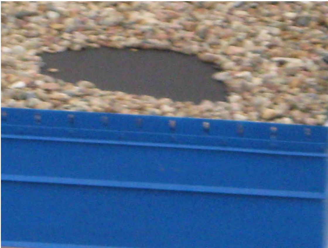
HAL 4/2009. PL-3. Bare spot in northwest corner of upper roof of the IHX building.
