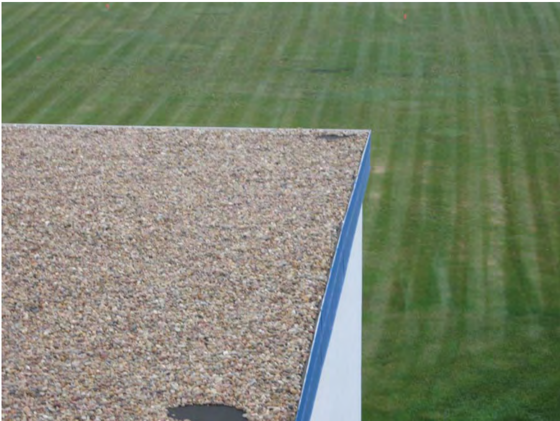
HAL 4/2009. PL-2. Two bare spots on the upper roof of the IHX building.
