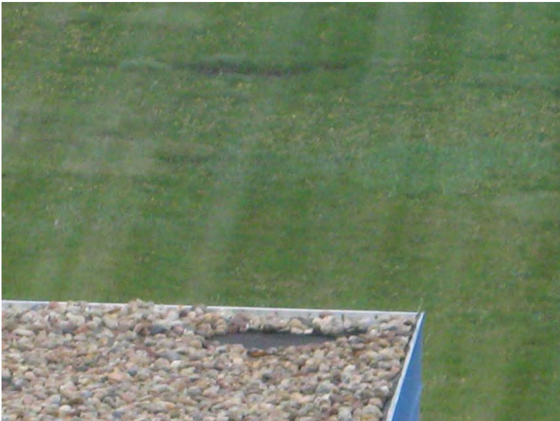
HAL 4/2009. PL-4. Bare spot in southwest corner of upper roof of IHX building.
