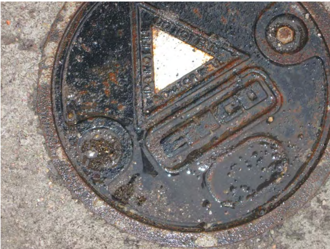
HAL 4/2009. PL-10. Well identification can be added to the white triangle on the well cap of the newly installed flush mount wells.
