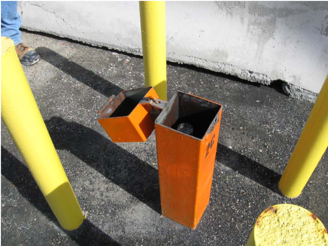
HAL 4/2010. PL-6. Broken hinge on the protective casing cap of monitoring well OBS-2C.
