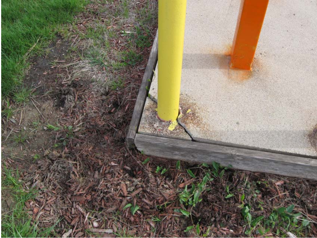
HAL 4/2010. PL-13. Northeast corner of the concrete pad at Wells OBS-8B and OBS-8C is cracked.
