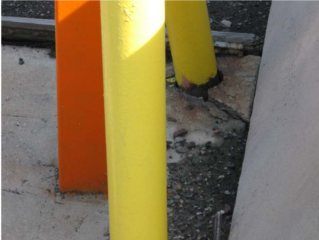
HAL 4/2010. PL-9. Concrete barrier east of monitoring wells OBS-2B2 and OBS-2C2. Concrete barrier has been pushed into the well pad. The wells are not damaged.
