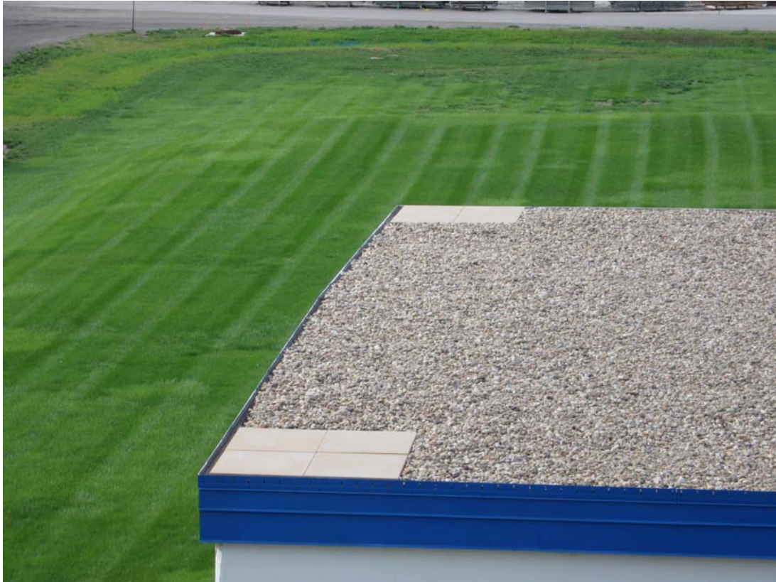
HAL 4/2010. PL-1. East corners of the upper roof of the IHX building.
