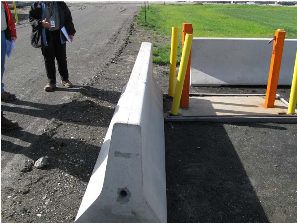
HAL 4/2010. PL-10. Concrete barrier east of monitoring wells OBS-2B2 and OBS-2C2 has been pushed into the well pad. The northeast corner of the well pad is cracked.
