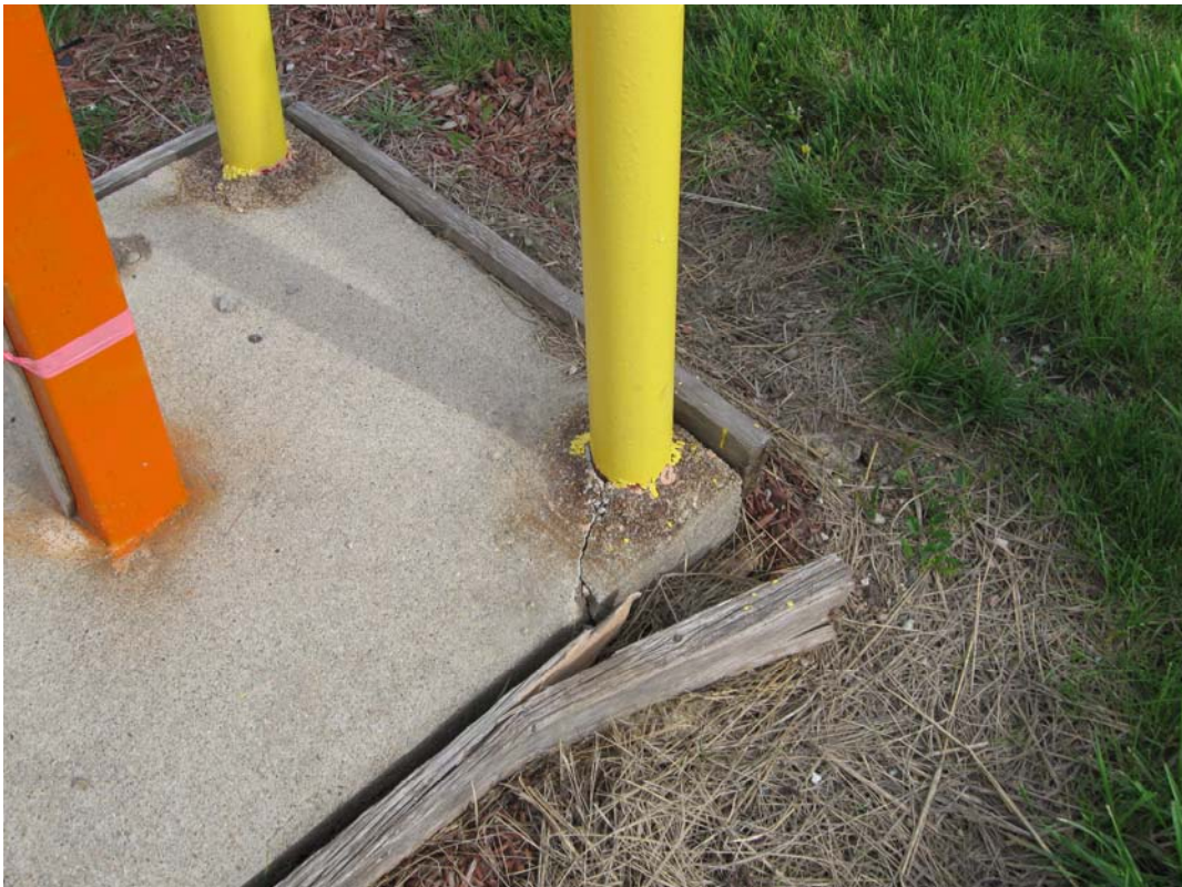
HAL 4/2010. PL-12. Southwest corner of the concrete pad at wells OBS-8B and OBS-8C is cracked.
