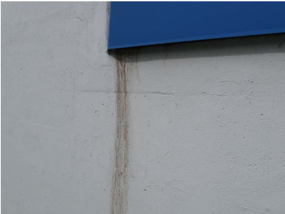
HAL 4/2012. PL-4. Water staining on east side of IHX building.
