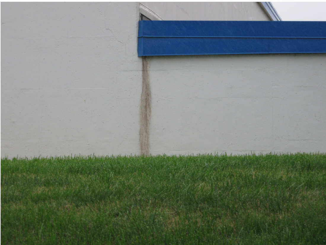
HAL 4/2013. PL-4. Stain on east side of IHX building.
