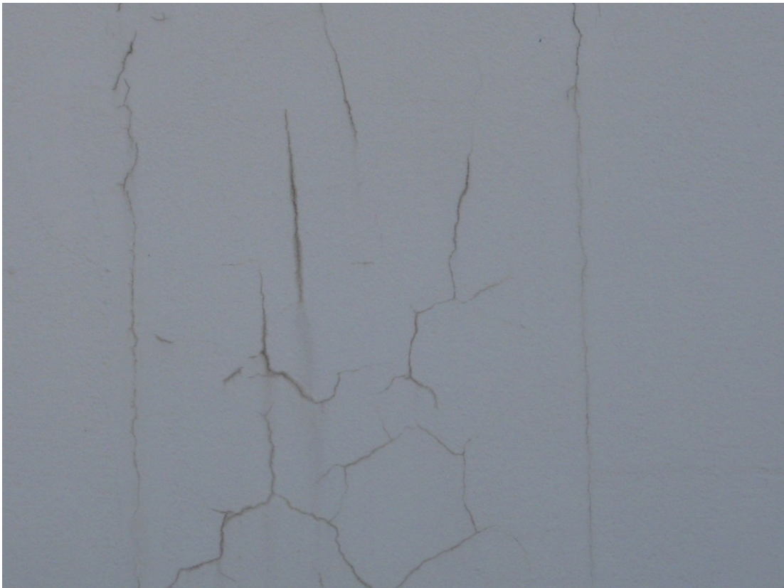
HAL 4/2014. PL-6. Surface cracks on north wall of IHX Building.
