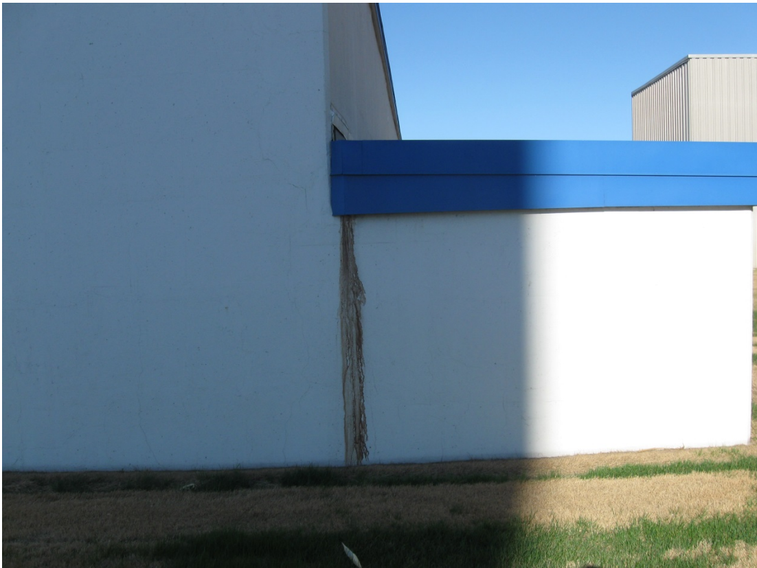
HAL 4/2014. PL-4. Water stain on east wall of IHX building.
