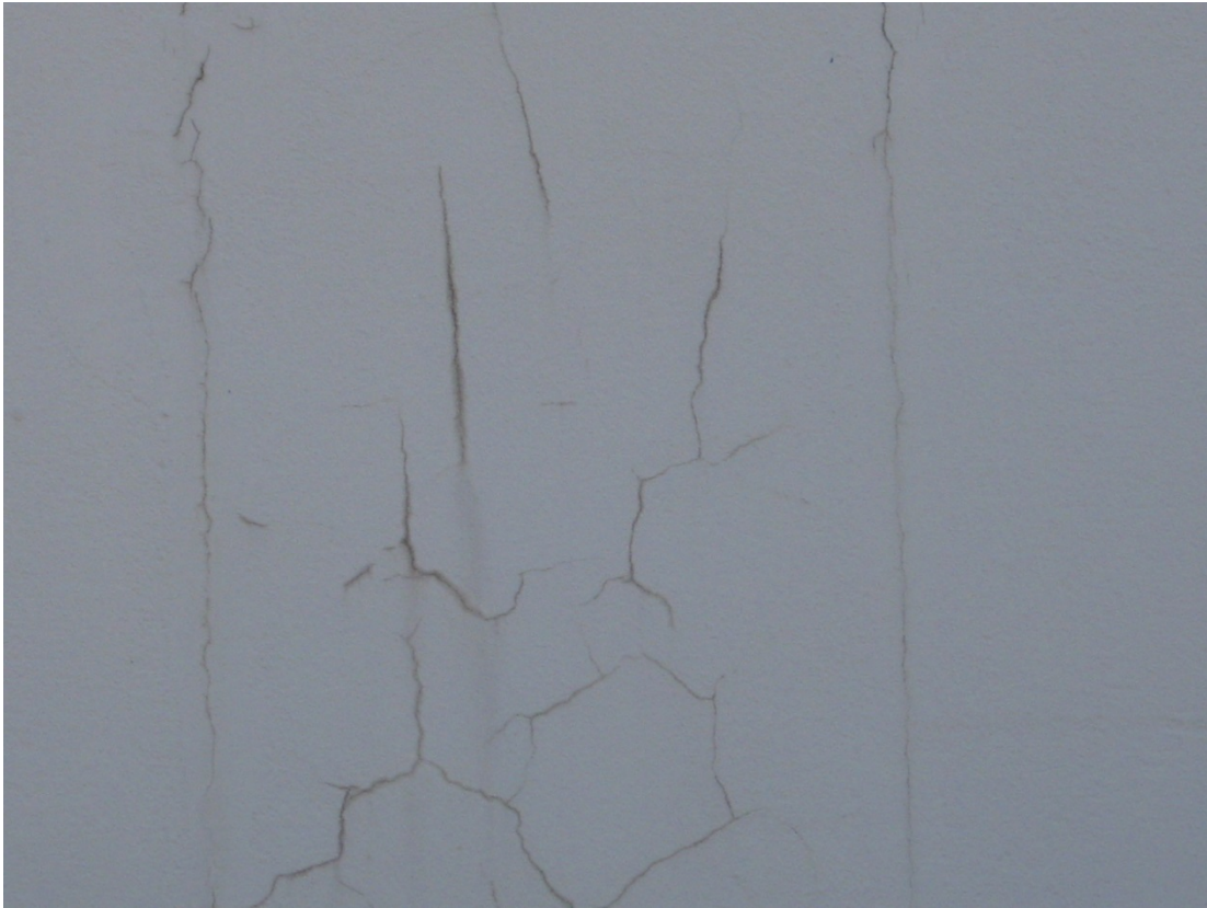
HAL 4/2014. PL-5. Surface cracks on north wall of IHX Building.
