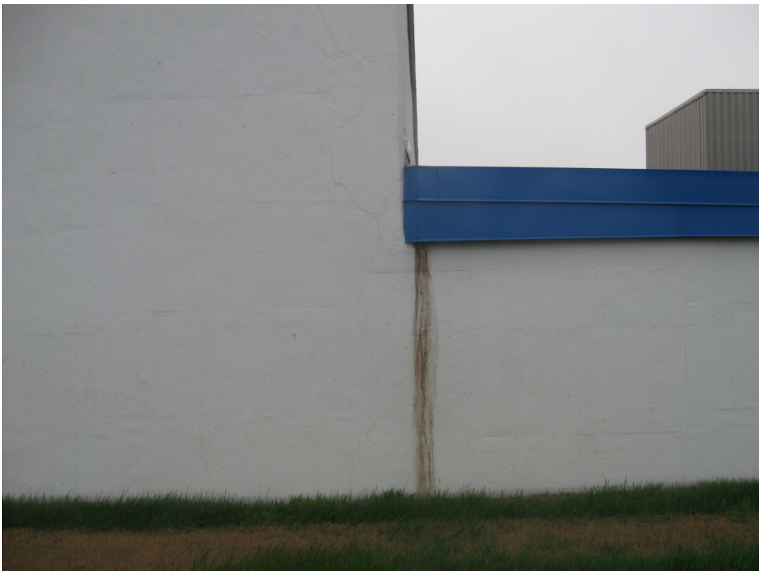
HAL 4/2015. PL-4. Water stains on east wall of IHX building.
