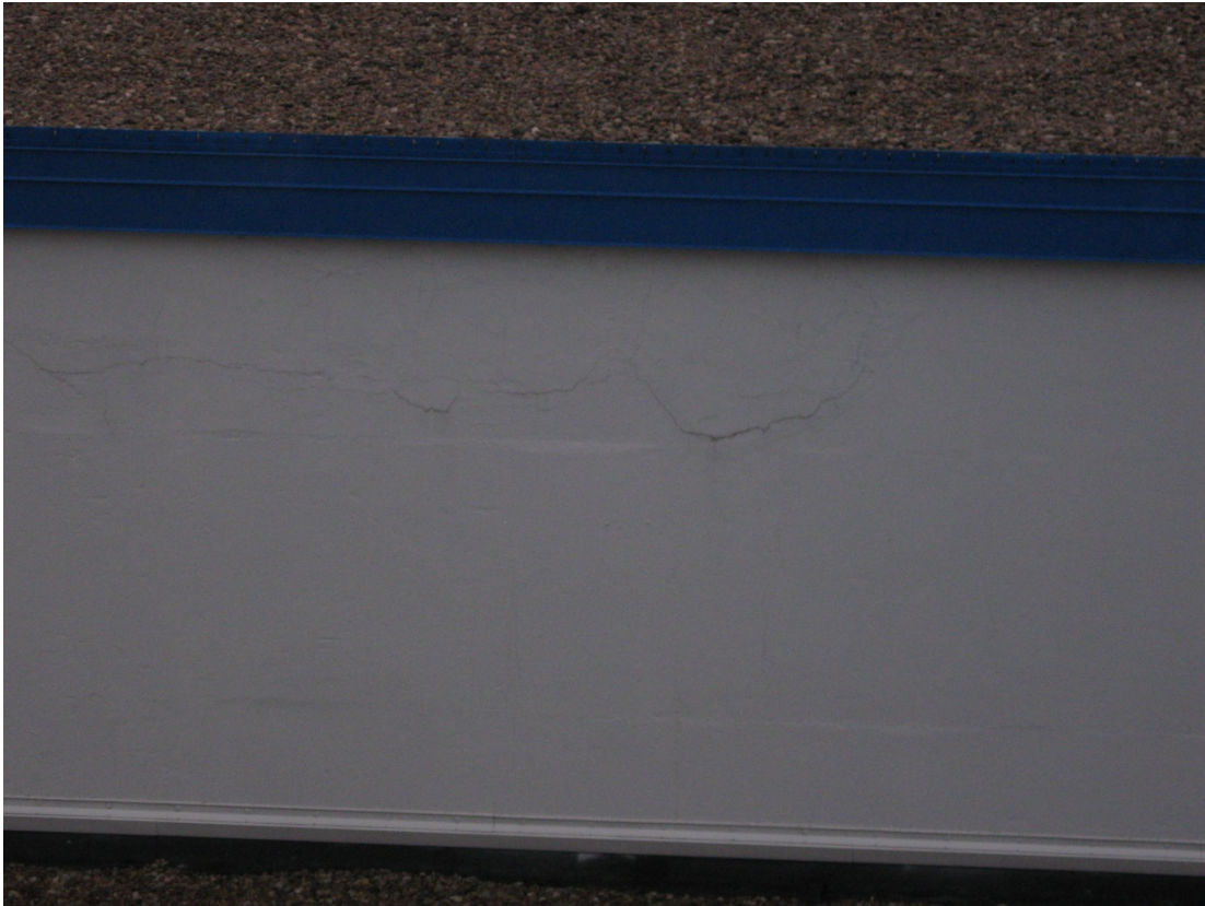
HAL 4/2015. PL-5. Surface cracks on north wall of IHX Building.
