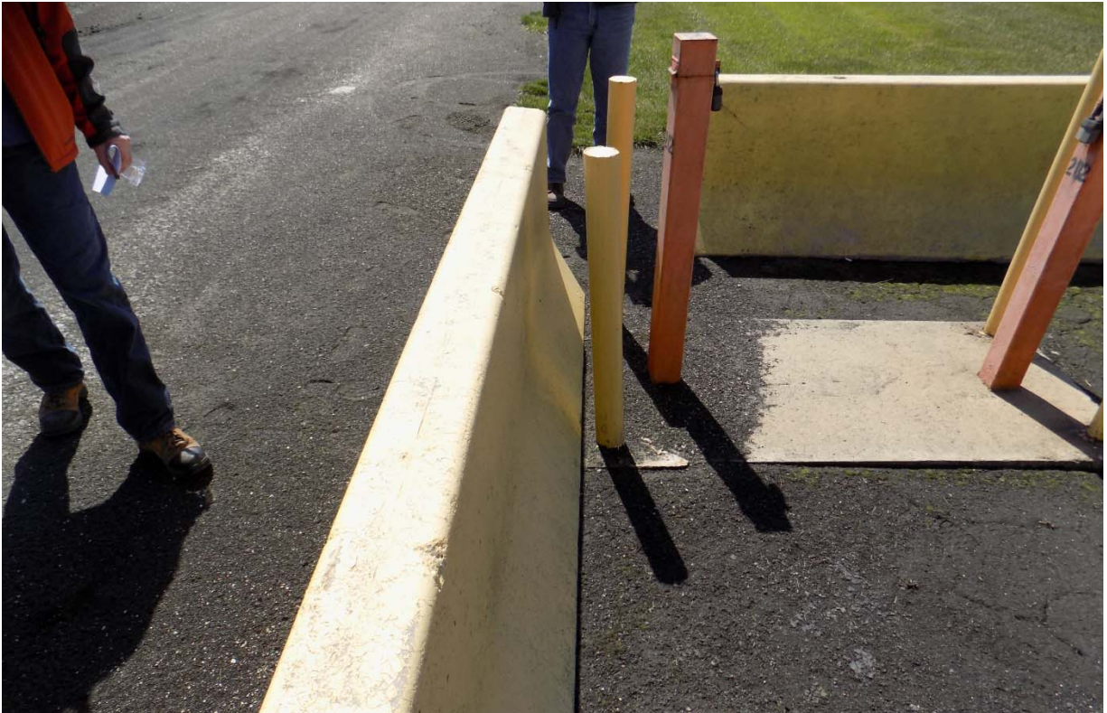
PL-13. Jersey Barrier Too Close to OBS-2 Well Pad
