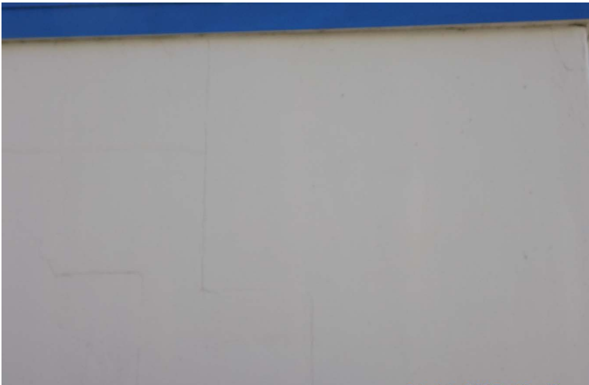
PL-6. Surface Cracks on North Wall of IHX Building
