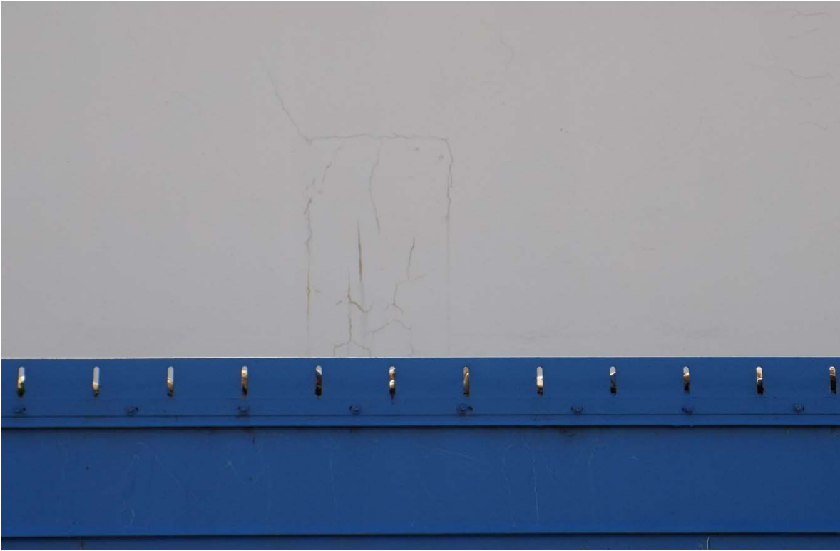
PL-5. Surface Cracks on North Wall of IHX Building
