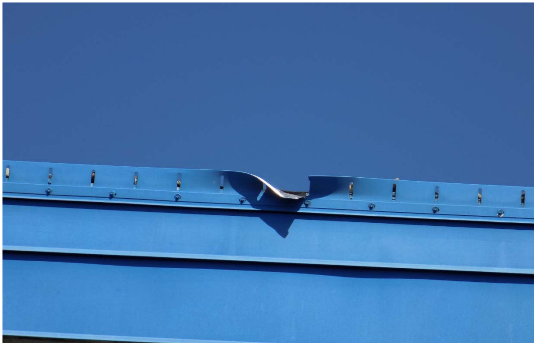
PL-4. Damaged Roof Edge
