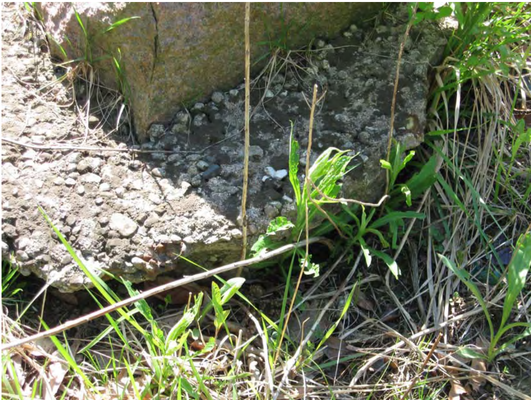
SAM 4/2010. PL-8. Erosion on Plot M north of the site marker is undercutting a corner marker.
