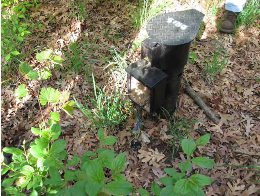
SAM 4/2010. PL-11. Back panel on protective casing at monitoring well DH-15 is missing. Wires are exposed to the public.
