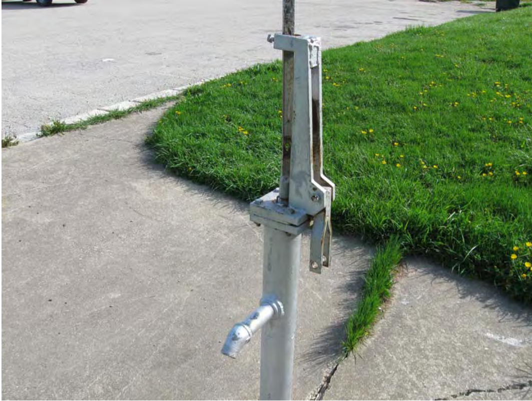
SAM 4/2010. PL-1. Public drinking water well at Red Gate Woods is inoperable because the handle has been removed.
