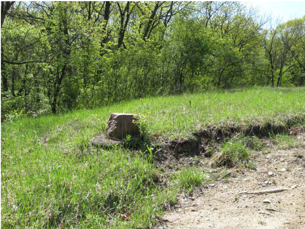
SAM 4/2010. PL-6. Erosion at Plot M undercutting the corner marker north of site marker.
