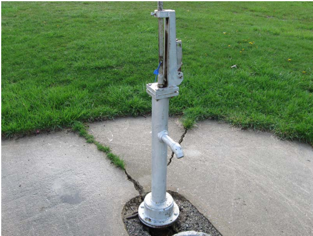
SAM 4/2011. PL-5. Disabled drinking water well at Red Gate Woods.
