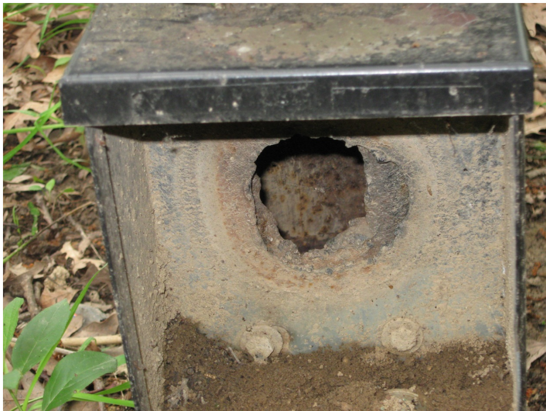
SAM 5/2012. PL-10. Hole in casing of monitoring well DH15.
