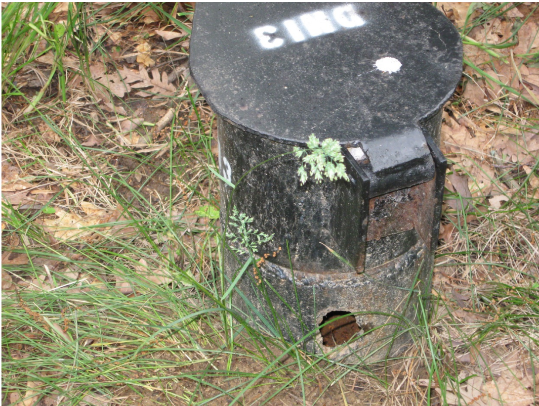
SAM 5/2012. PL-12. Hole in casing of monitoring well DH13.
