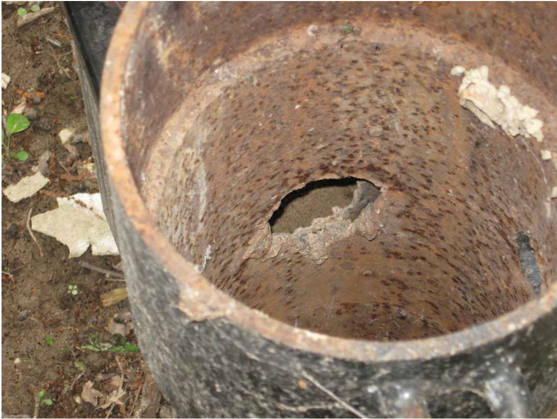
SAM 5/2012. PL-11. Hole in casing of monitoring well DH15.
