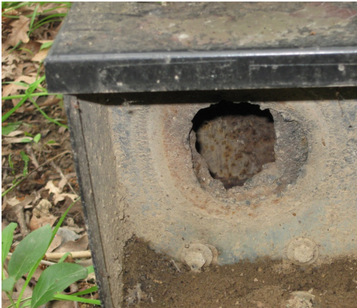
SAM 4/2013. PL-12. 2012 photo of monitoring well BH-15.
