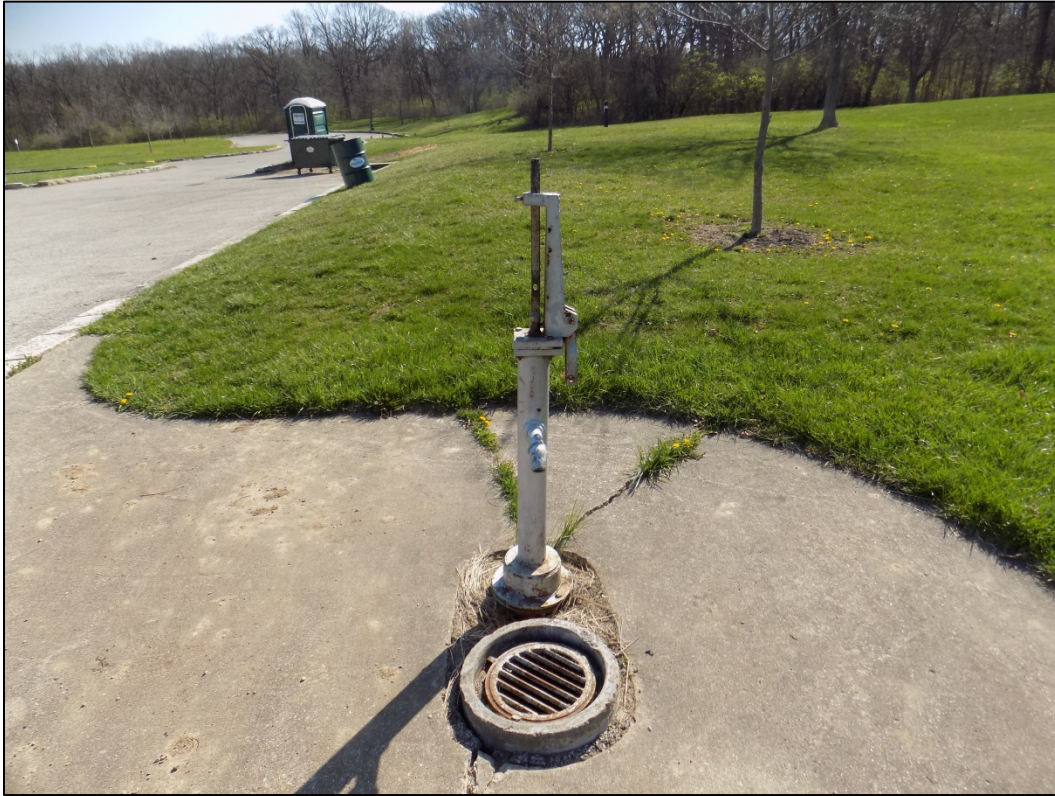
PL-1. Handle Removed from Picnic Area Well 5160 in Red Gate Woods Area
