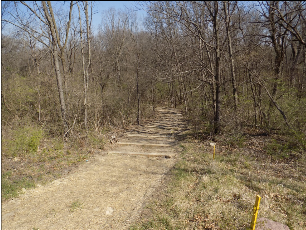
PL-7. Looking North down Path with New Timbers Installed to Reduce Erosion
