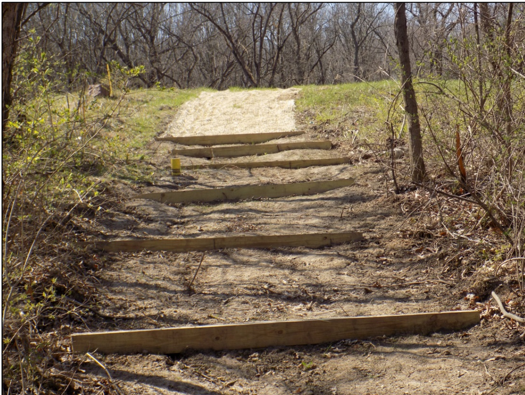
PL-8. Looking South at Erosion-Control Timbers Installed in Footpath Leading to Plot M
