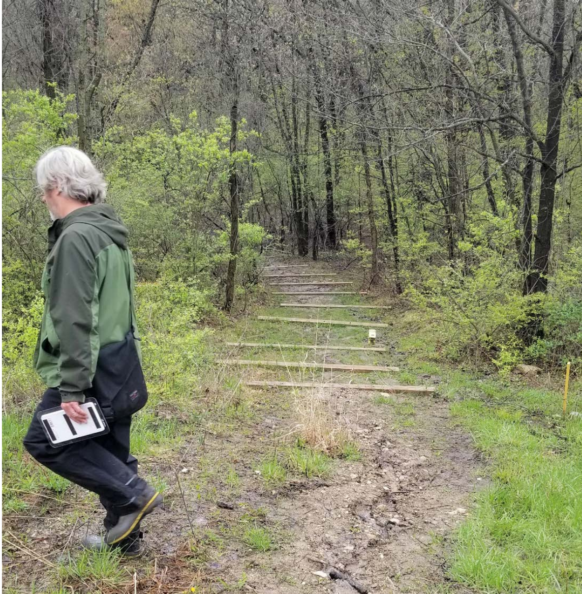
Figure 1.3 North view of timber steps installed along northeast path at Plot M.
