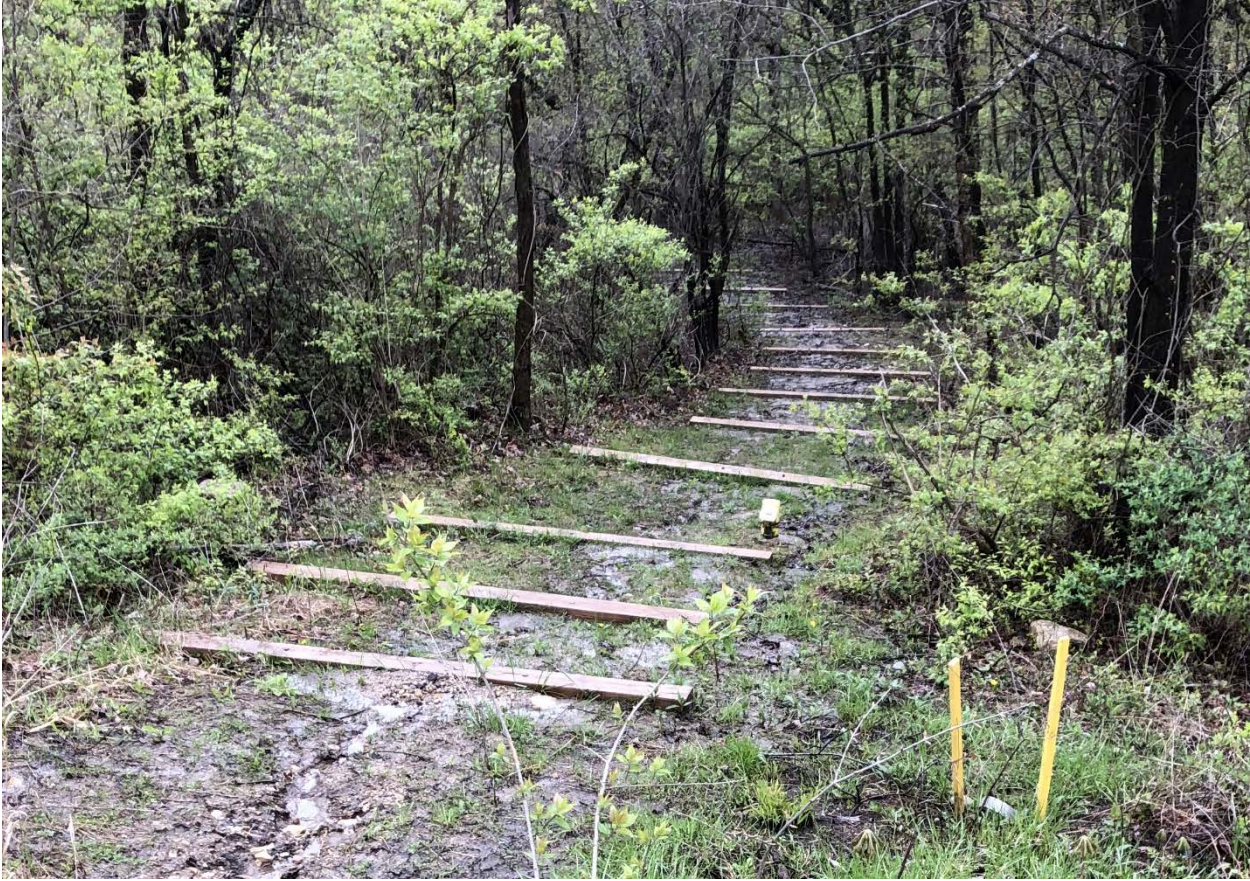
Figure 1.2 Northeast view of timber steps installed along the path at Plot M.
