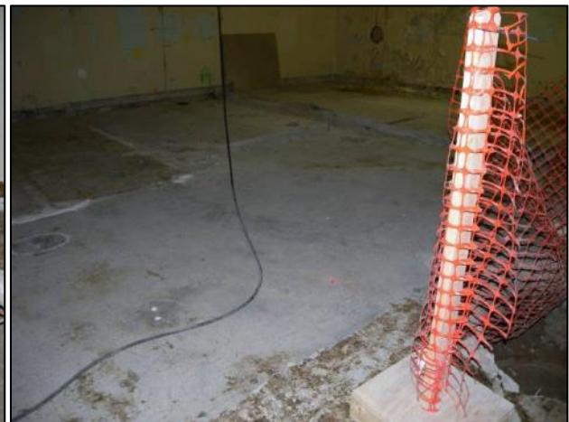
Figure C-29. T Building Room 63 View J
