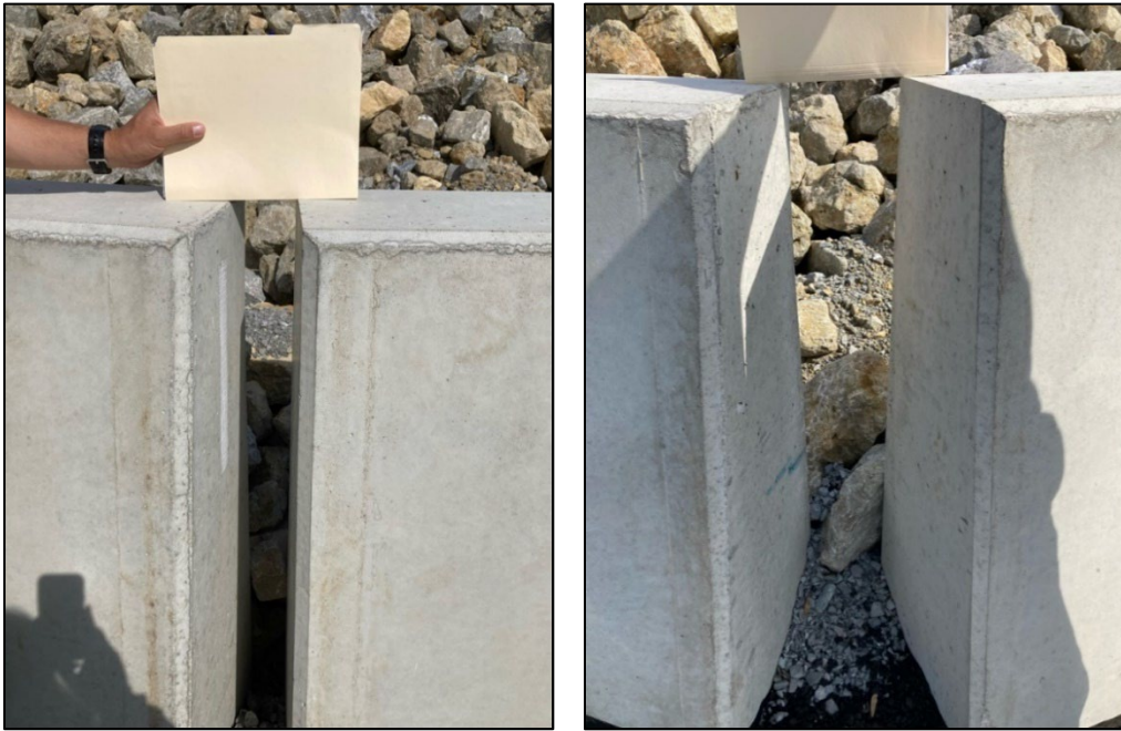
Figure 2. Examples of Spacing Between Protective Jersey Barriers
