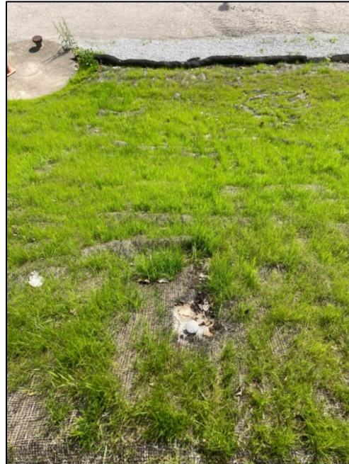
Figure 7. Small Erosion Near Base of Hillside
