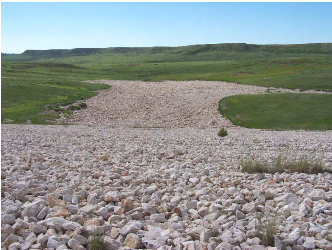
EDG 6/2008. PL-8. Main drainage channel viewed from the top of the tailings embankment.
