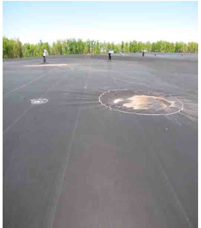
Previous subsidence repair in southeast portion of interim cap.
