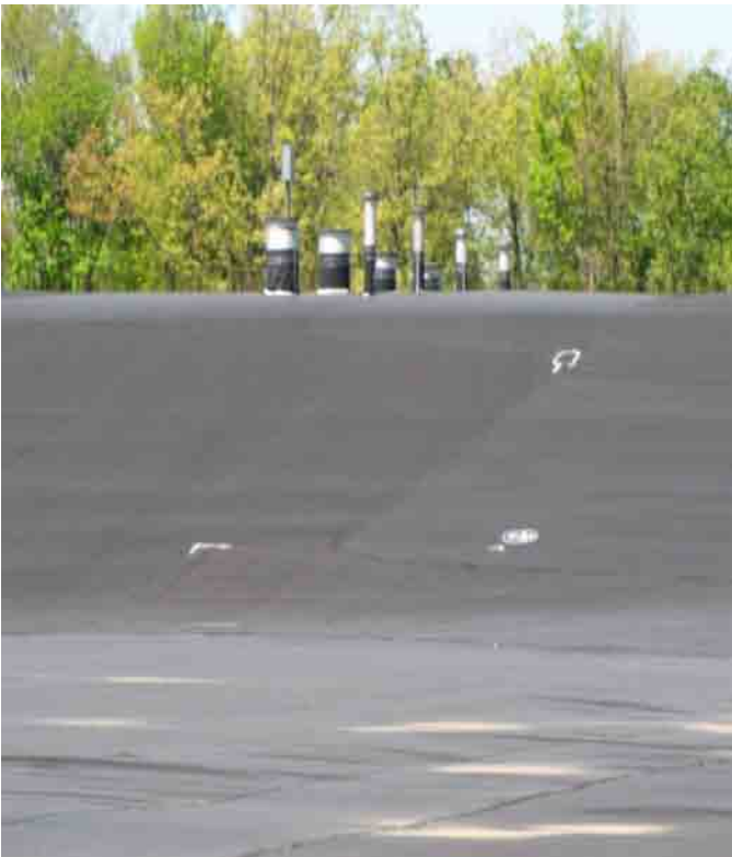
Top of the former leachate storage facility; viewing tank access extensions that are cathodically protected.
