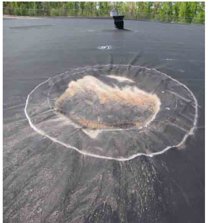
Previous subsidence repair in southeast portion of interim cap.
