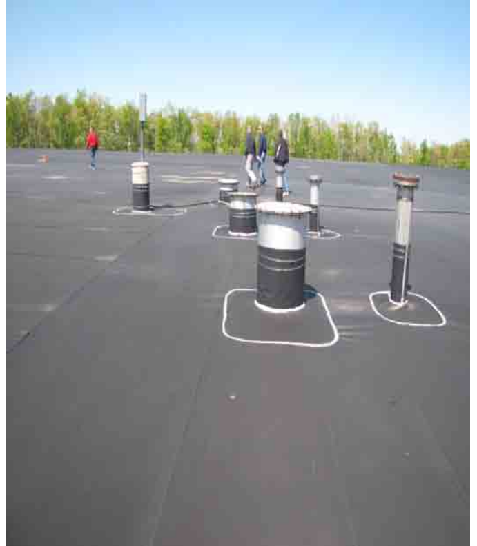
Commonwealth access points to 20,000 stainless steel tanks and cathodic protection system.
