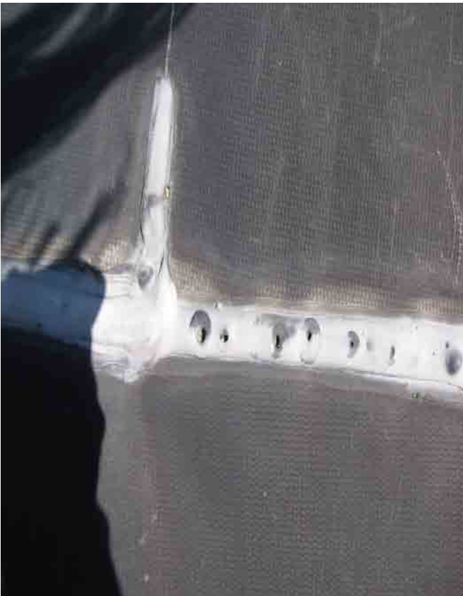
White extrusion weld exhibiting bubbling and holes.
