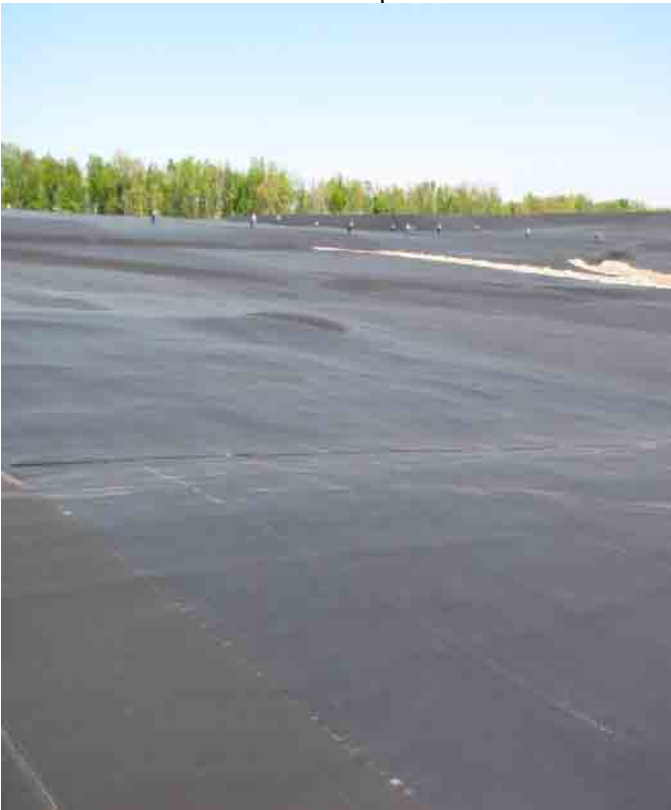
View of interim cap from southeast portion of liner; y-channel on right.
