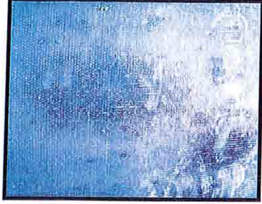
Deterioration on Surface of Liner (typical)
