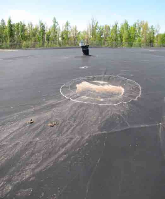
Previous subsidence repair in southeast portion of interim cap.
