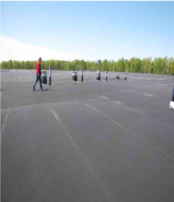
Top of previous leachate storage facility; Commonwealth access point to 20,000 stainless steel tank below.
