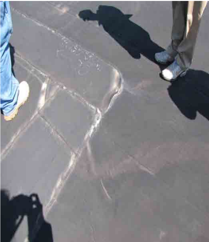
Corner of interior diversion berm of interior cap. Note evidence of flow from corner.
