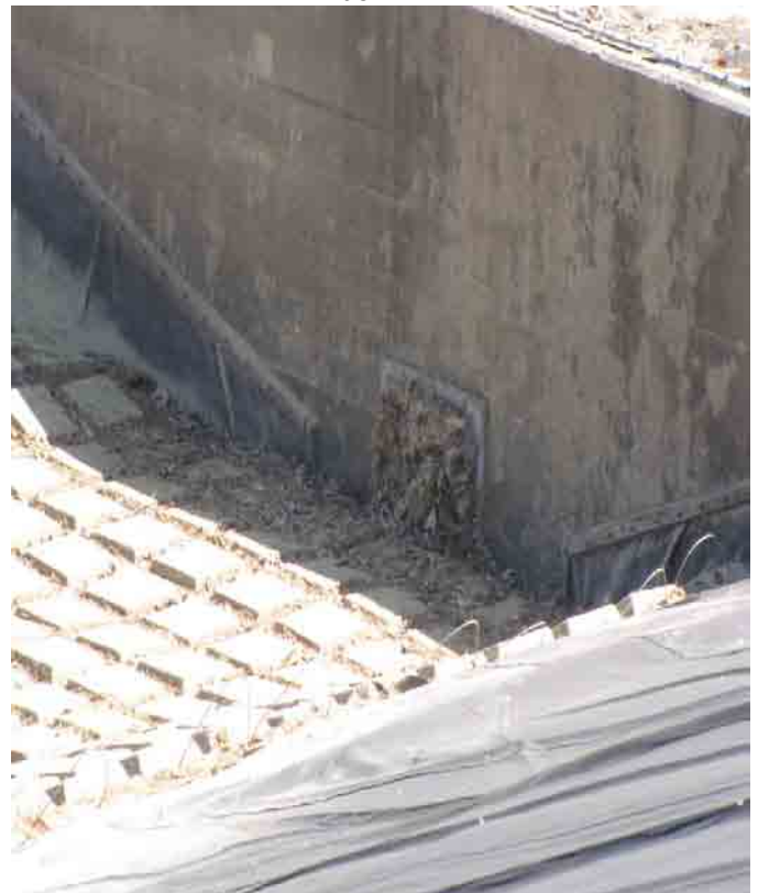
Close-up of grate into NE corner piping at Eastern end of north channel.
