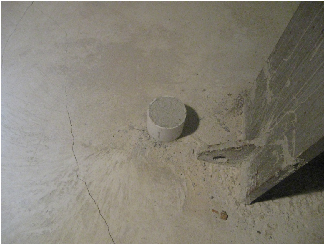
BON 8/2013. PL-8. Floor drain filled with cement.
