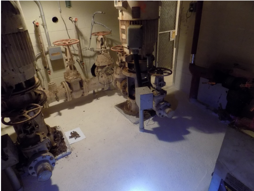
PL-5. Contaminated oil-stained rust at base of condensate pump in basement of containment building
