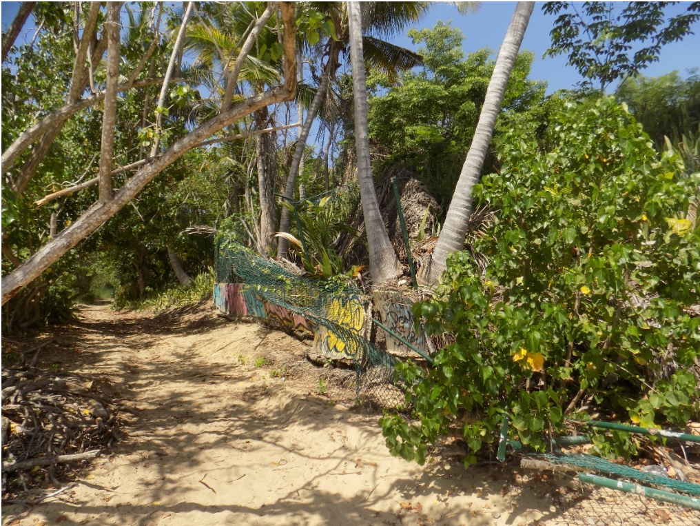
PL-9. Damaged security fence
