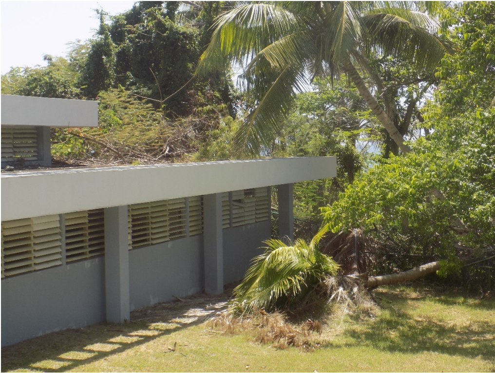
PL-10. Downed tree on roof of training center
