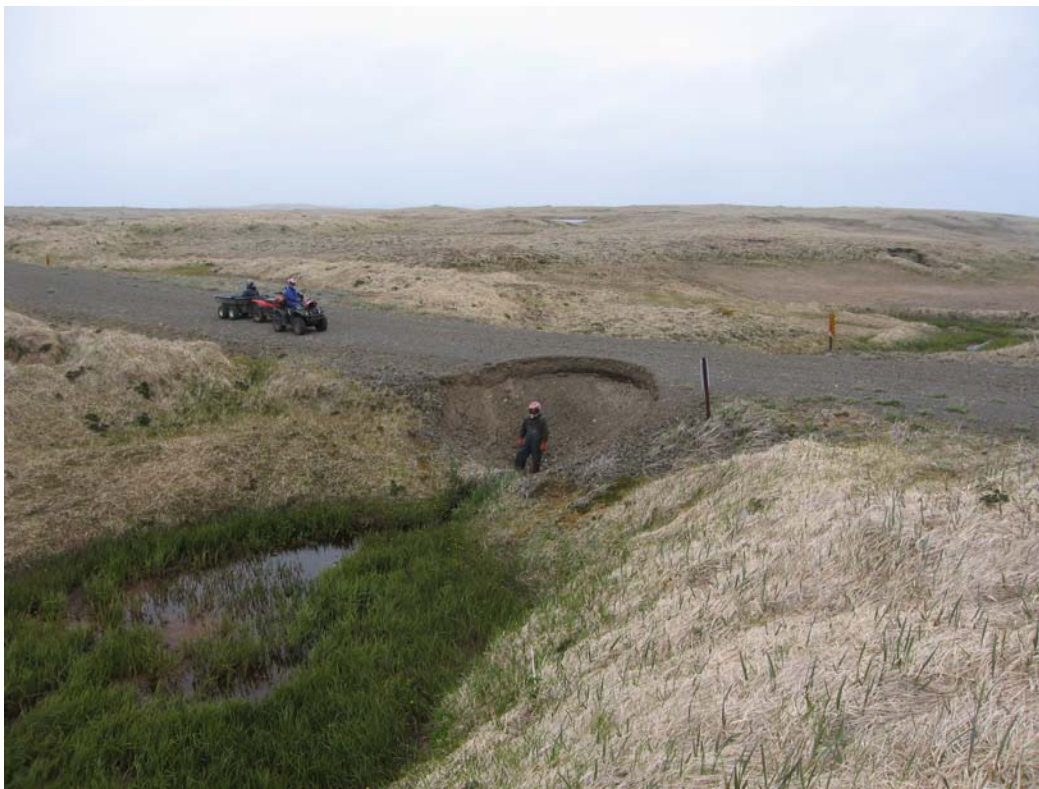
Figure 7. Infantry Road Partial Washout near MM 4
