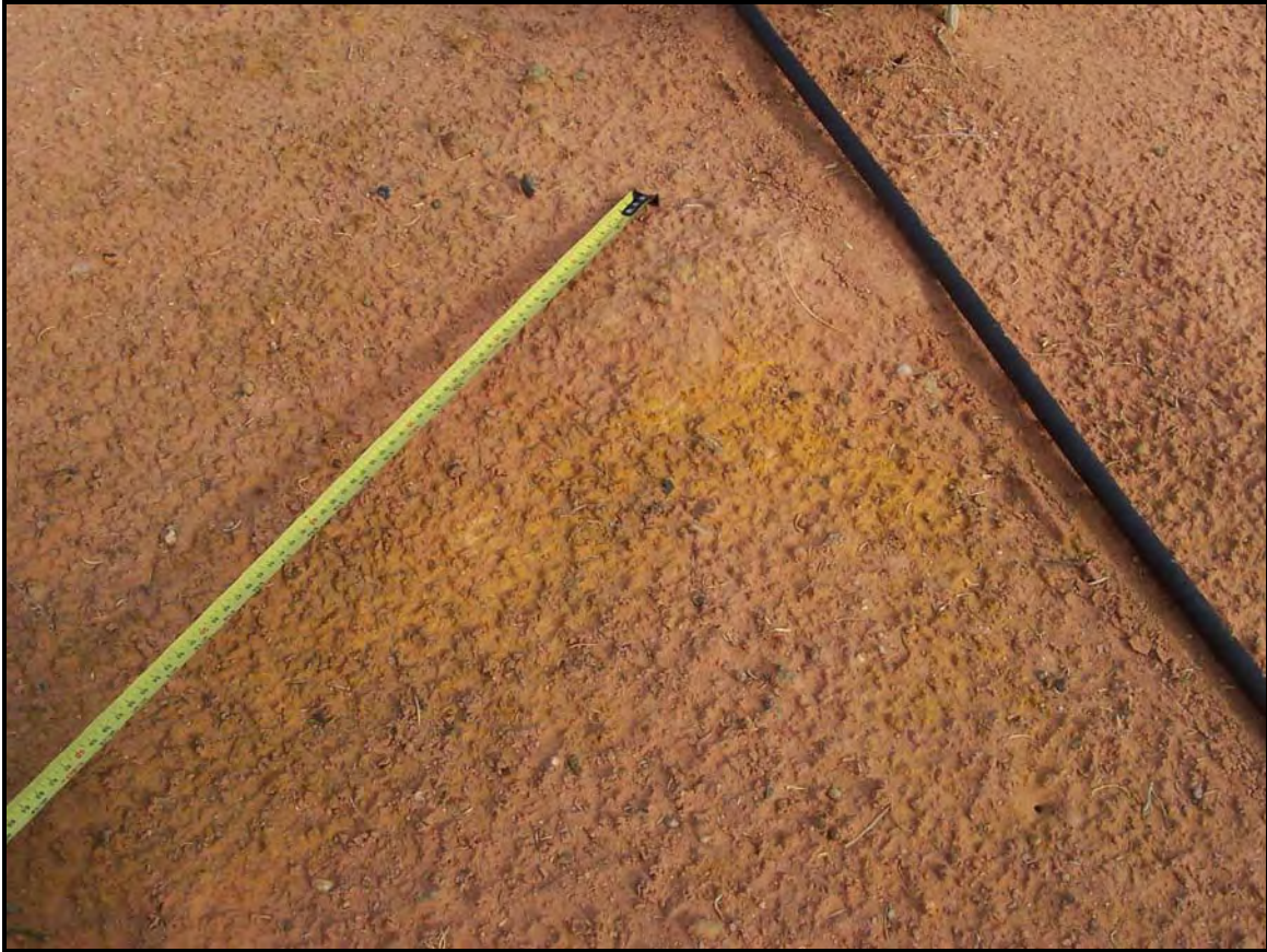
Close-up of yellow stain in former evaporation pond area.
