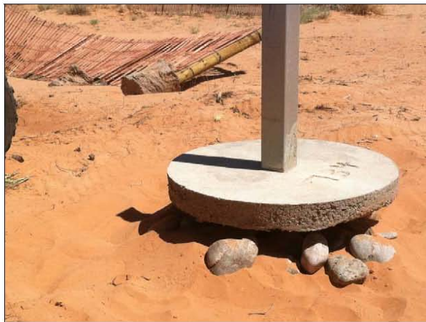
Erosion at well 0734. Note the fence post in the background.
