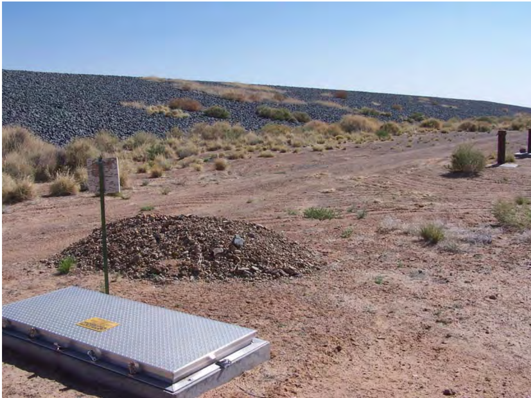
TUB 4/2008. PL-2. Vegetation encroachment on the south side slope of the disposal cell (reference photograph taken from extraction well 1107).
