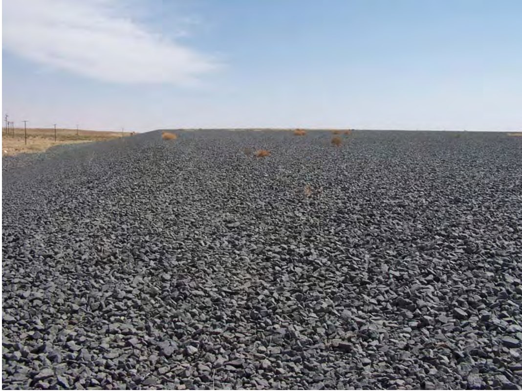
TUB 4/2008. PL-1. The cell top and side slope along the northwest side of the disposal cell.
