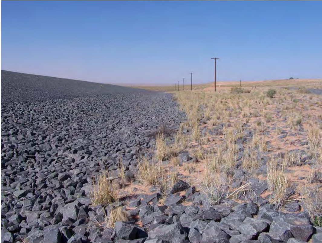
TUB 4/2008. PL-3. View of drainage ditch along the northwest side of the disposal cell.
