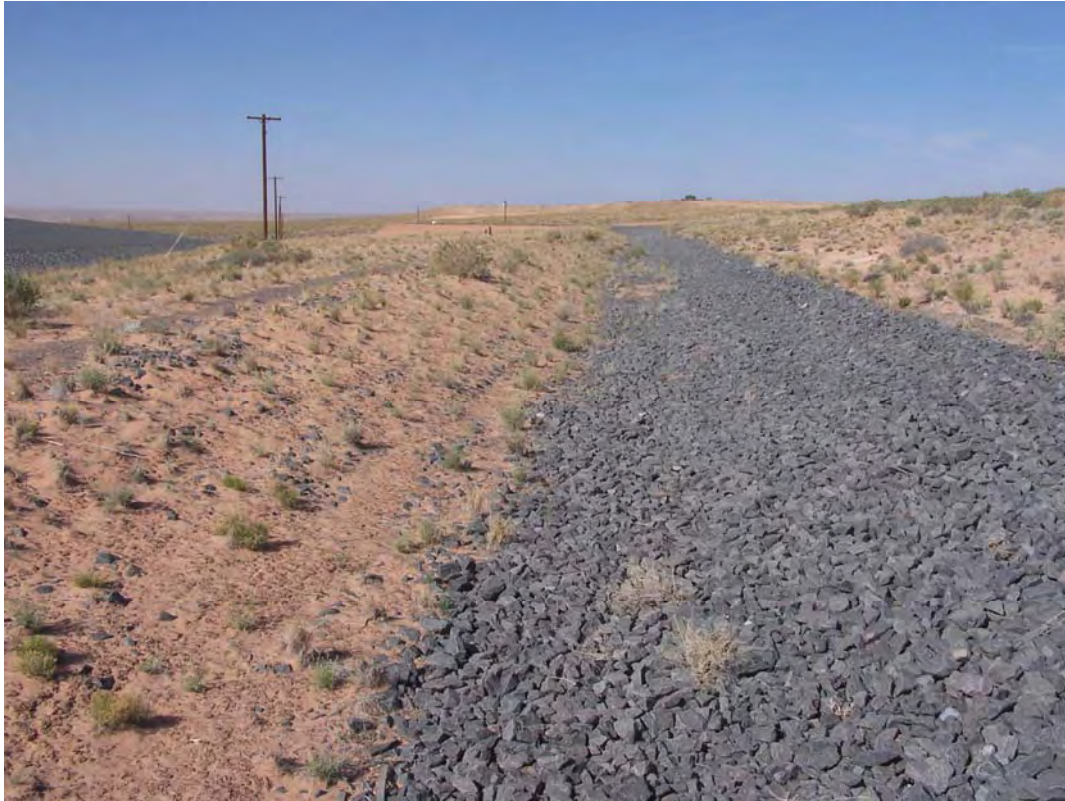
TUB 4/2008. PL-5. Vegetation encroachment in windblown sand accumulating on the south bank of the diversion channel (repeat photograph taken from the footbridge).
