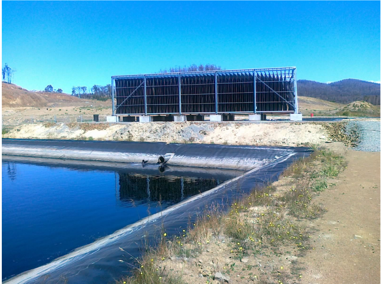
Figure 10. Typical WAIV Process Installation
