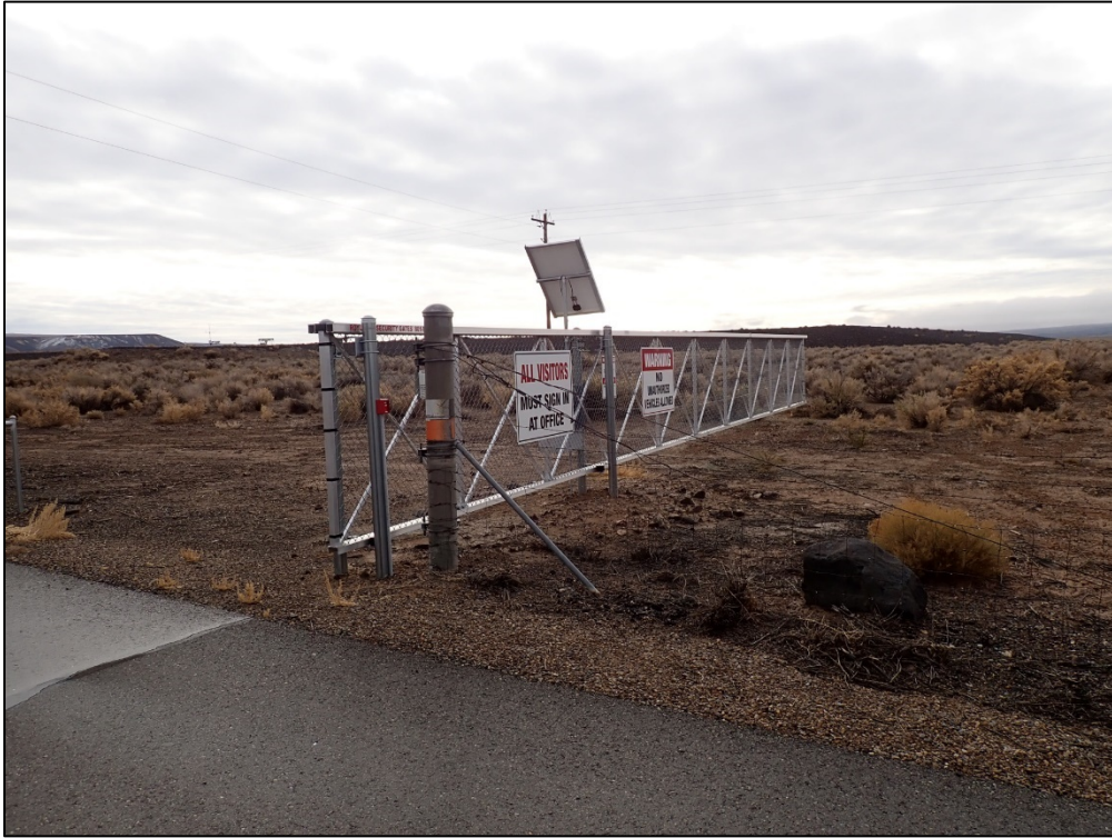
PL-1. Solar-Powered Site Entrance Gate
