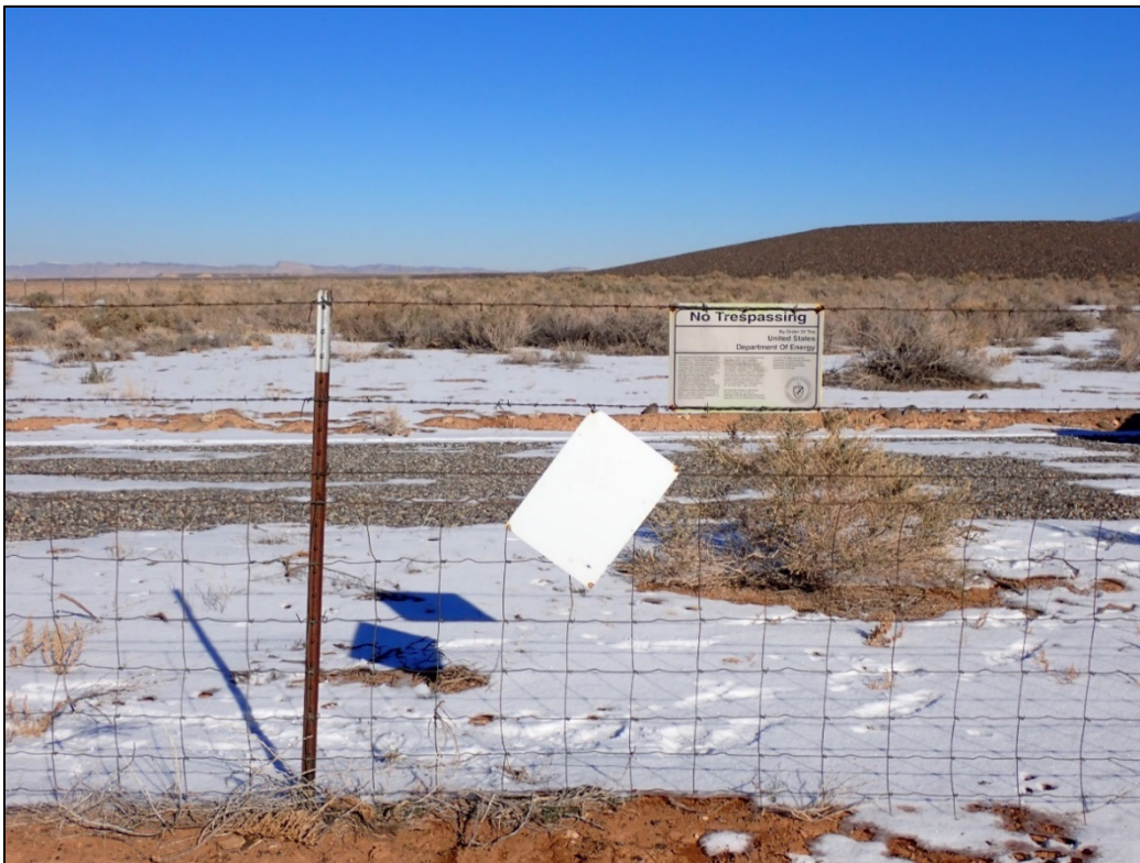
PL-4. Partially Detached Perimeter Fence Sign
