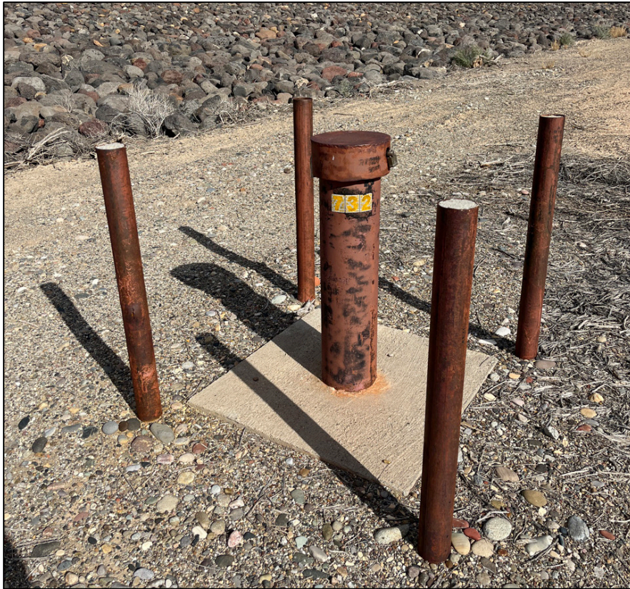
PL-5. Monitoring Well 0732
