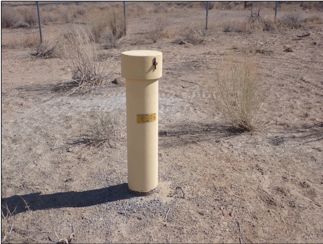
PL-7. Faded Identification Numbers on Monitoring Well 0176
