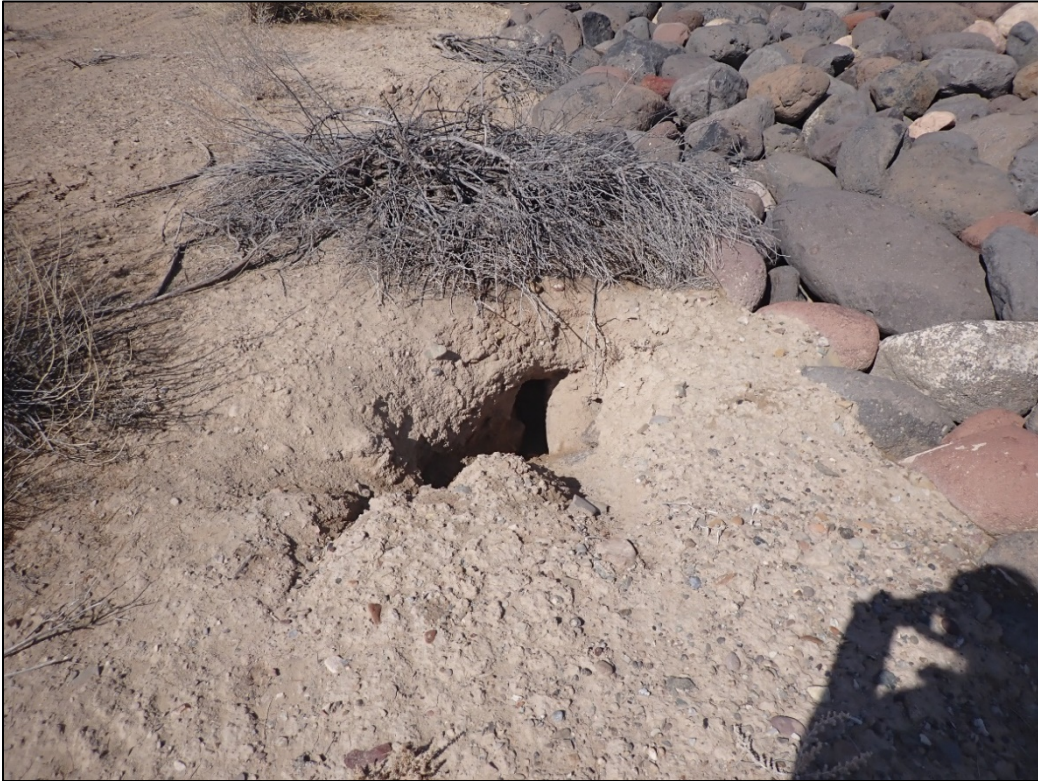
PL-11. Soil Piping on Edge of Rock Apron
