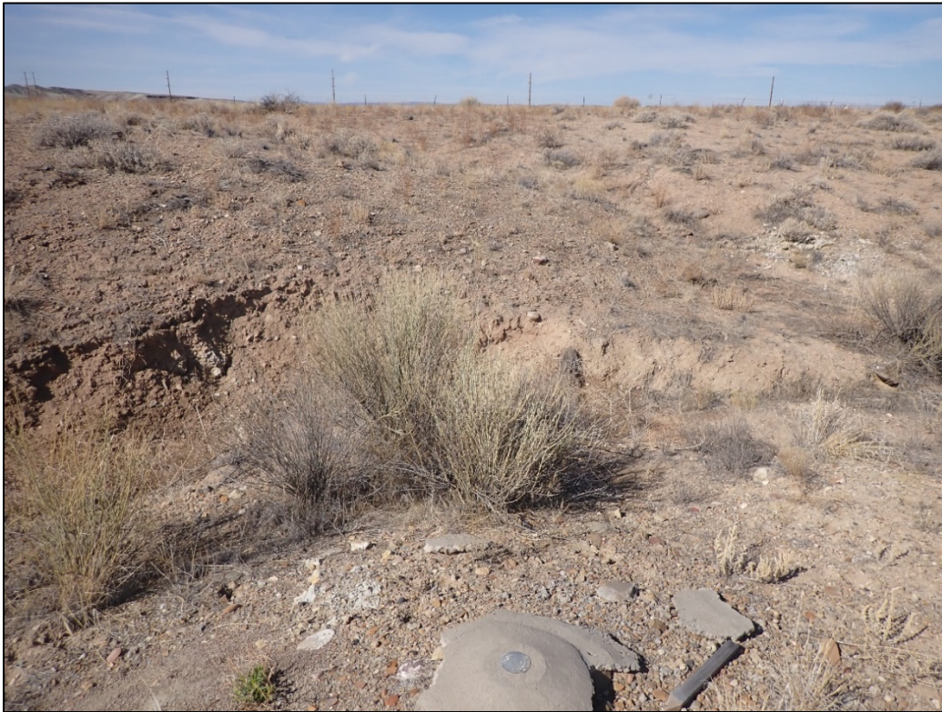
PL-5. Cracked and Spalled Concrete Around Survey Monument SM-2
