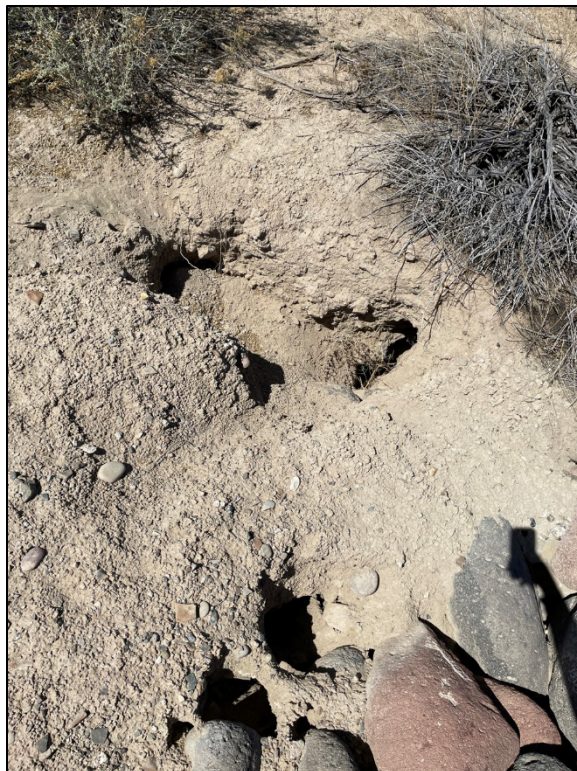
PL-6. Erosion at South Corner of Disposal Cell
