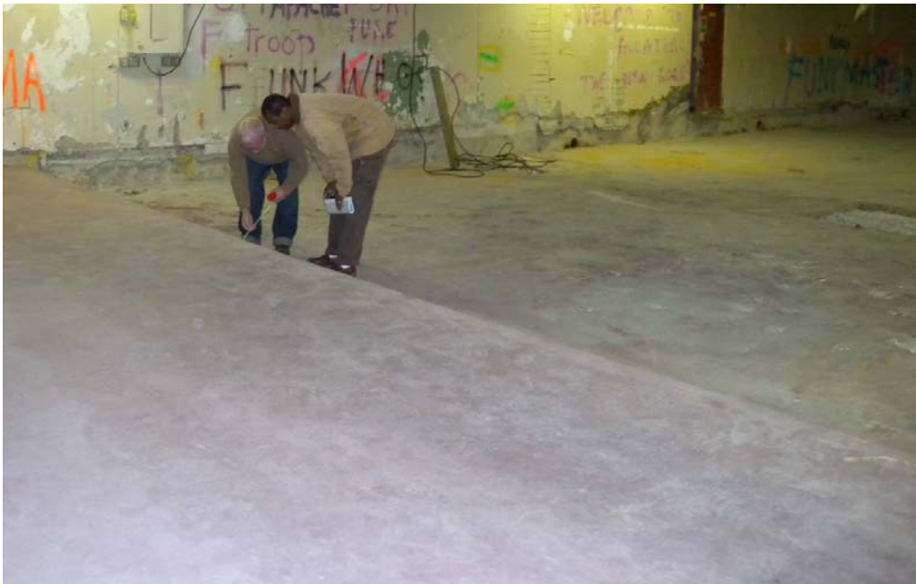
Figure 10. Art Kleinrath and Anthony Campbell examine edge of red concrete slab in T Building areas where penetration of concrete floor is prohibited without prior approval
