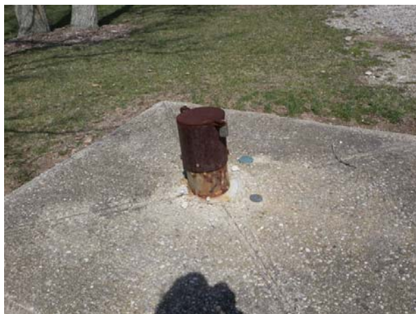
Figure 12. Well 0124 offsite condition during 2010 IC assessment
