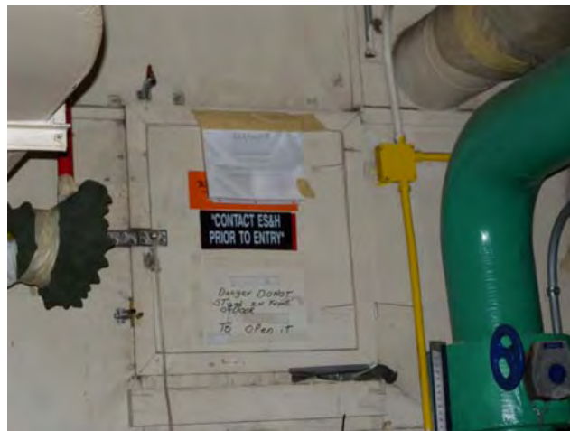
T Bldg. Room 99 - Access door to airshaft with special ICs leading to west head house
