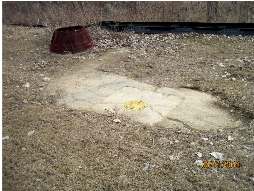
Figure 12. Area Around Well 0346 is Still Affected by Storm Water Runoff
