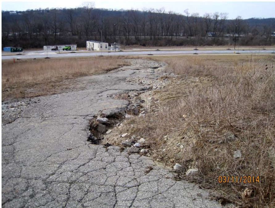
Figure 23. Erosion of Roadway East of LM Trailers, Caused by Clogged Drain. The Roadway is Used to Access Monitoring Wells
