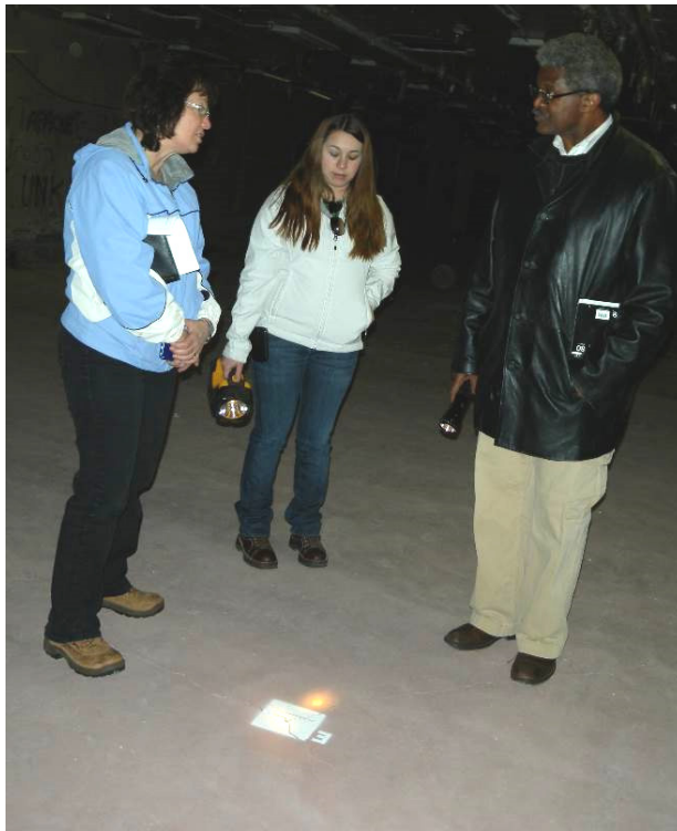
Figure 19. Gwen Hooten and Shelly Vigil, LM; and Larry Kelly, EMCBC Examine Cracks During Walkdown in T Building, April 15, 2014
