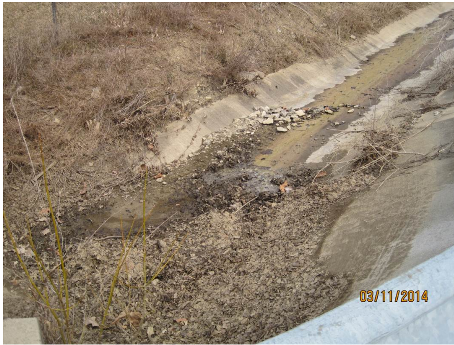
Figure 22. Debris Clogging Drain Uphill East of OU-1
