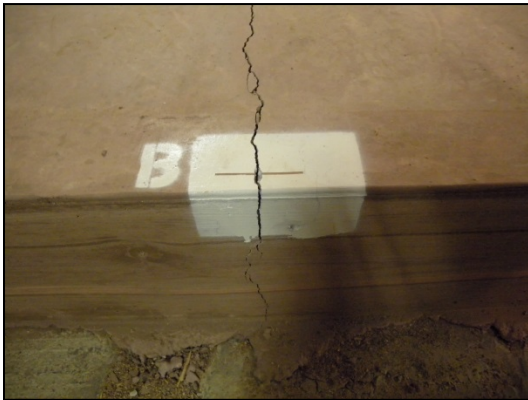
Monitoring point B
