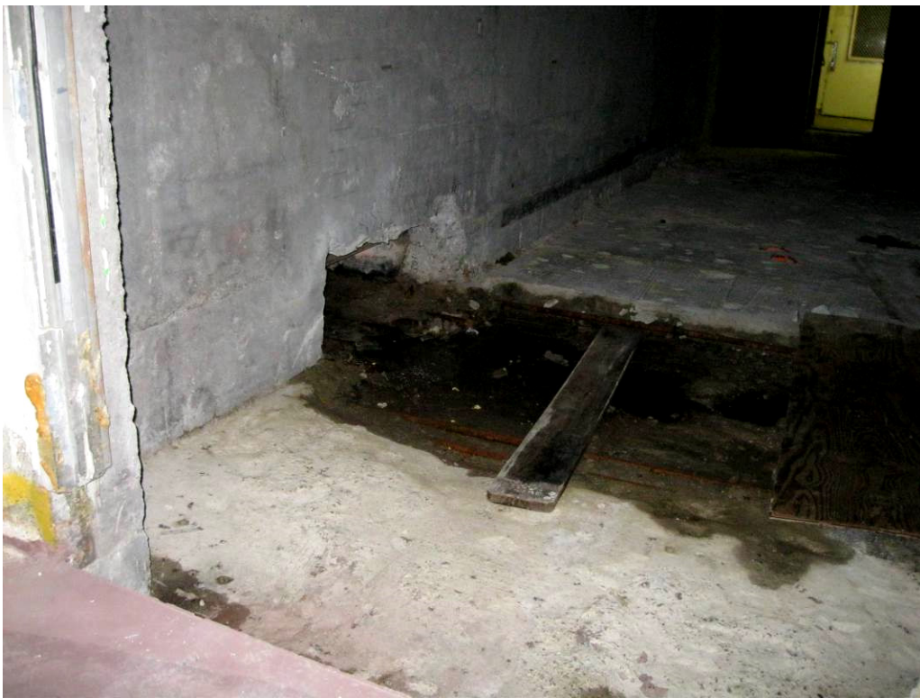
Figure 21. Water on the Floor of Room 57 in T Building in March 2014
