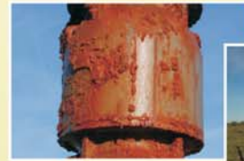
Iron-fouling on pump and pipe
