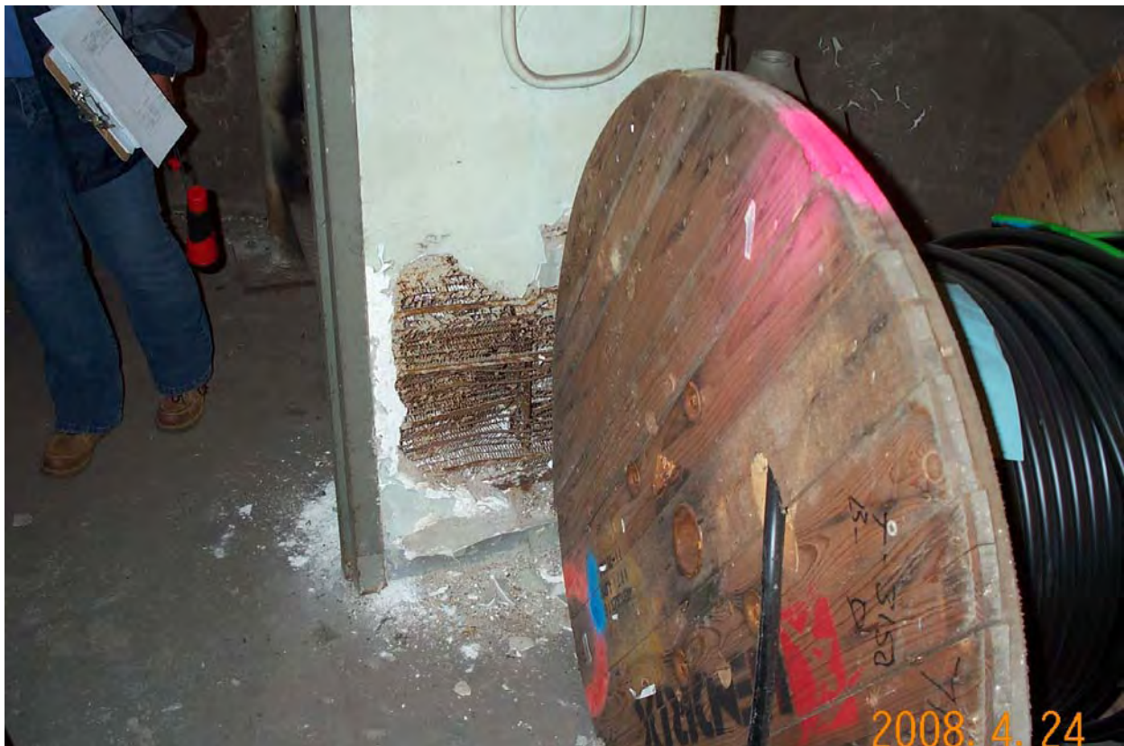
PIQ 4/2008. PL-6. Damage to Walls by Cable Spools, 56-foot level.
