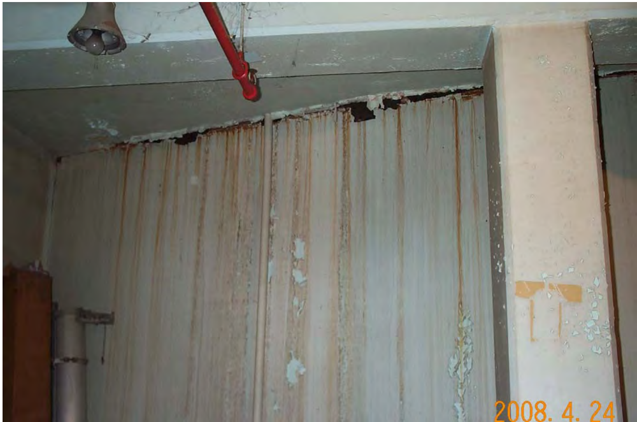
PIQ 4/2008. PL-7. Water corrosion along seam of wall in Room B-1, 79-foot level.
