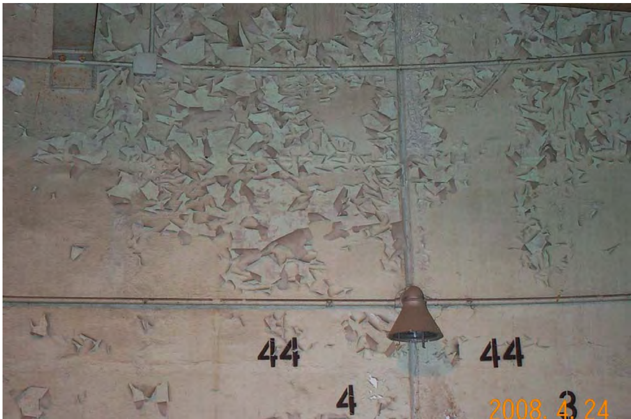
PIQ 4/2008. PL-4. Peeling Pain, 56-foot level.
