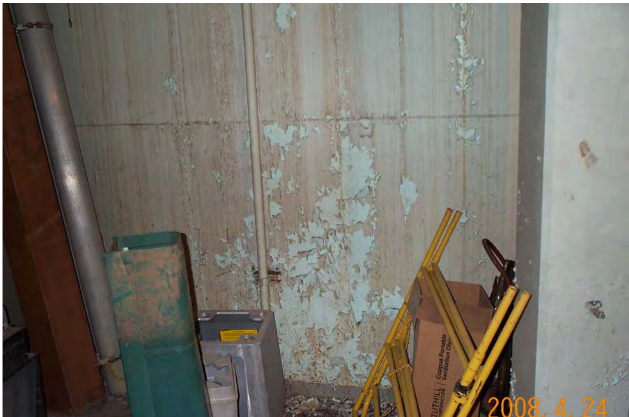
PIQ 4/2008. PL-8. Peeling paint, Room B-1, 79-foot level.
