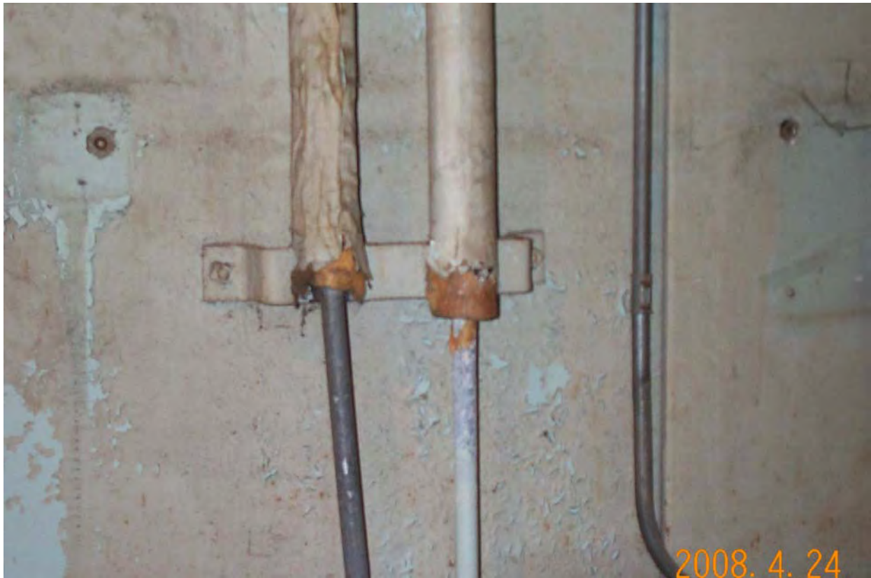
PIQ 4/2008. PL-9. Worn insulation, 79-foot level.
