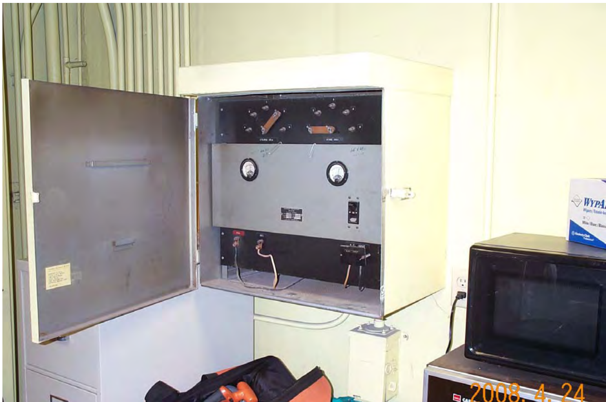
PIQ 4/2008. PL-10. Rectifier control panel, 100-foot level.
