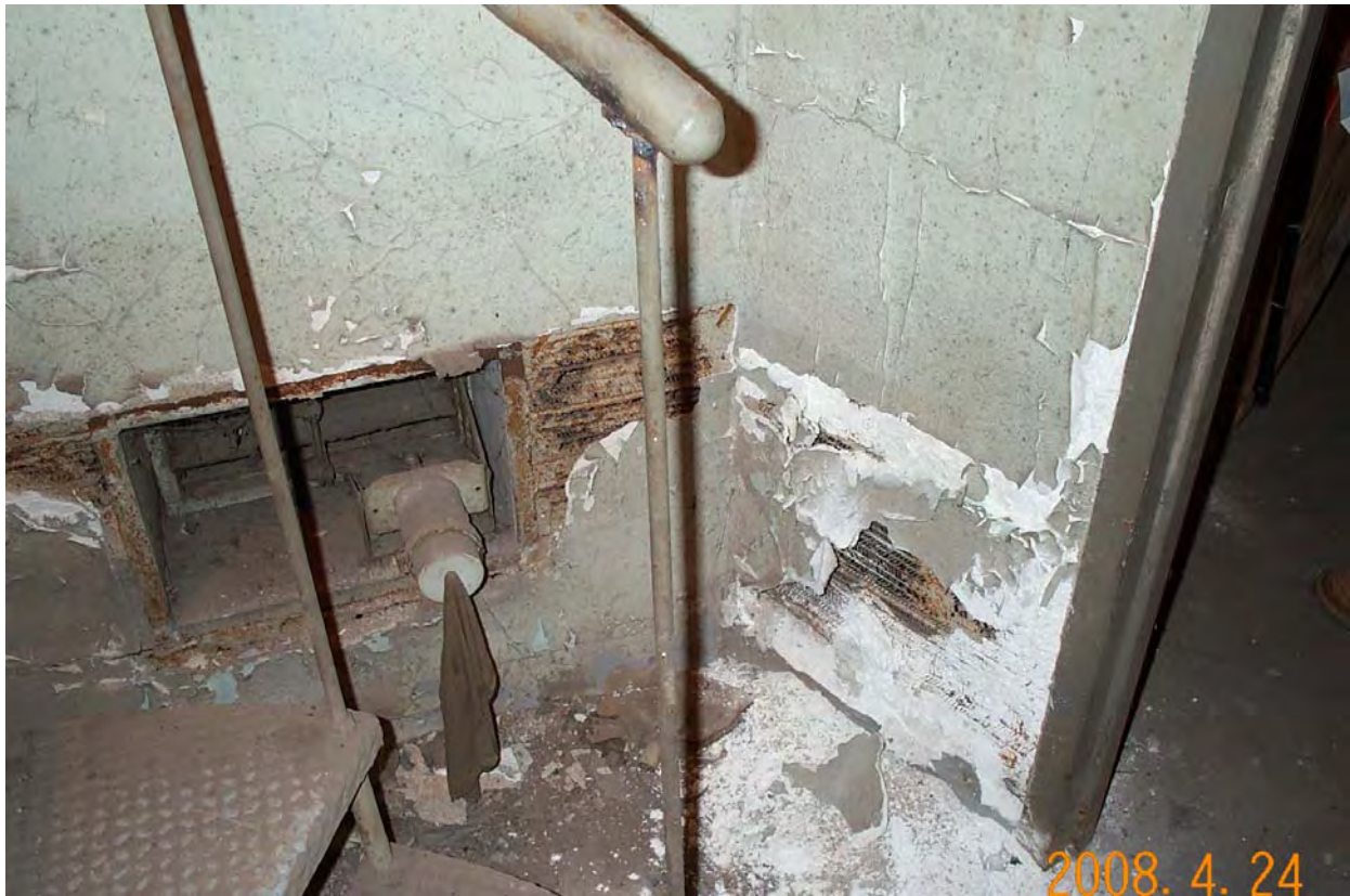
PIQ 4/2008. PL-5. Water Damage, Base of Spiral Stairs, 56-foot level.
