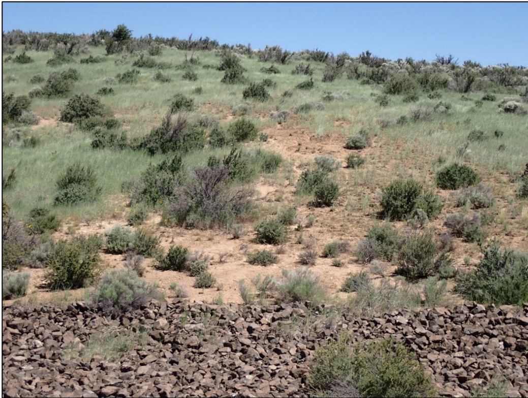
PL-12. Erosional Features on North Slope of Disposal Cell
