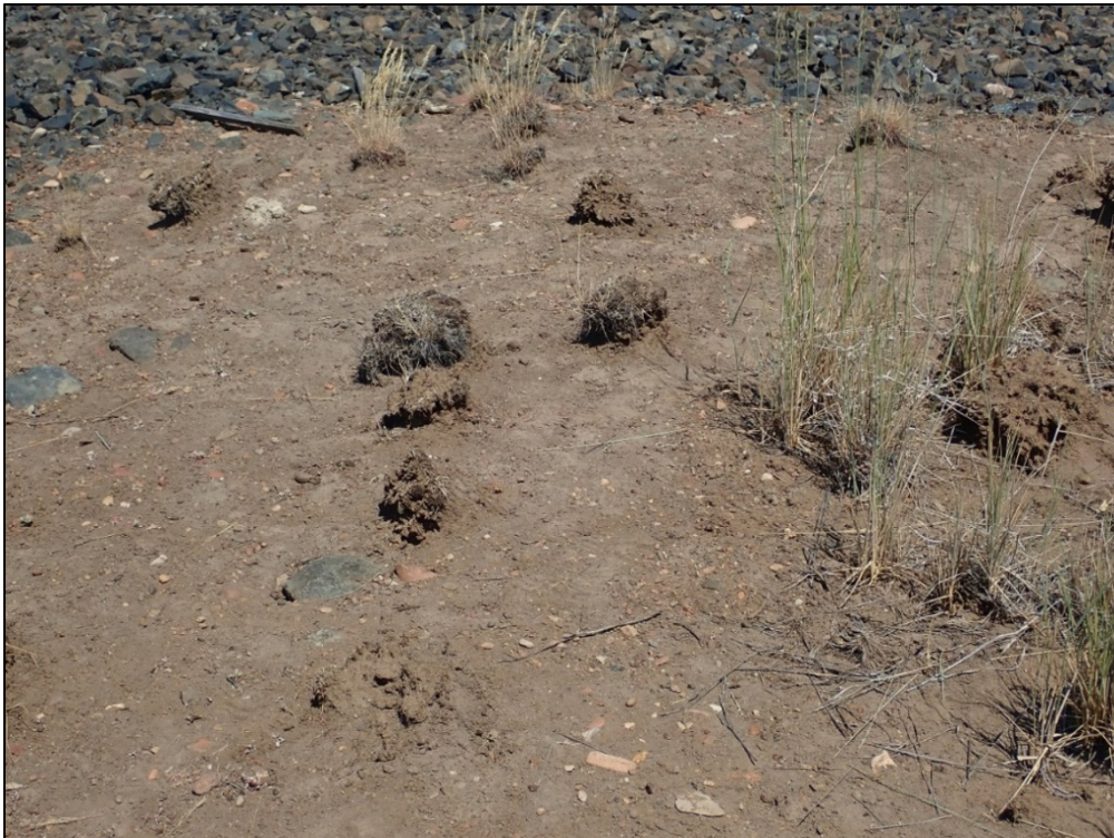
PL-7. Windblown Erosion on Northwest Corner of the Disposal Cell
