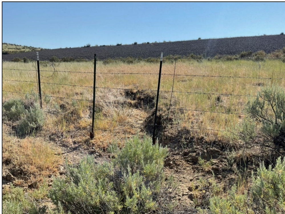
PL-9. Headcutting at Apron Toe Drain 3
