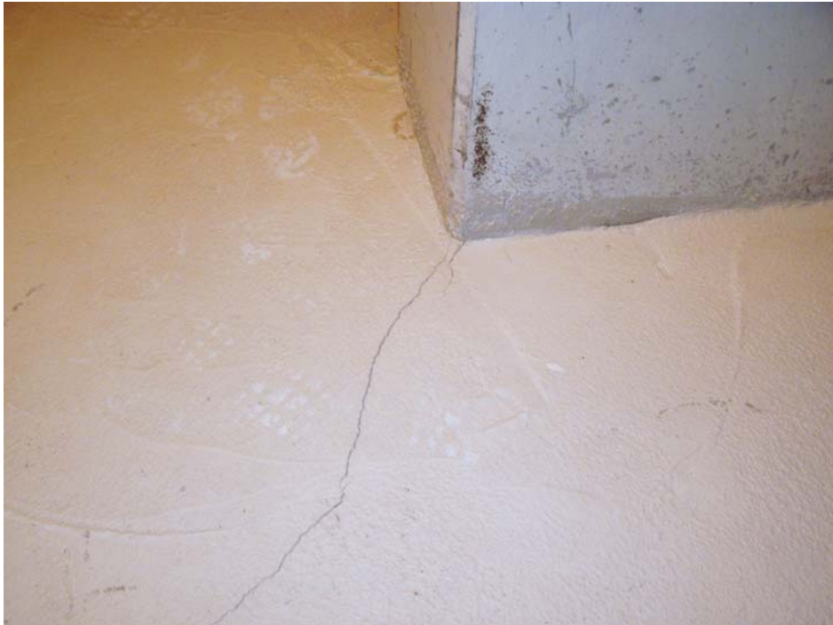
Figure 8. Basement Level – Surface Cracks in Concrete Cover (Typical)
