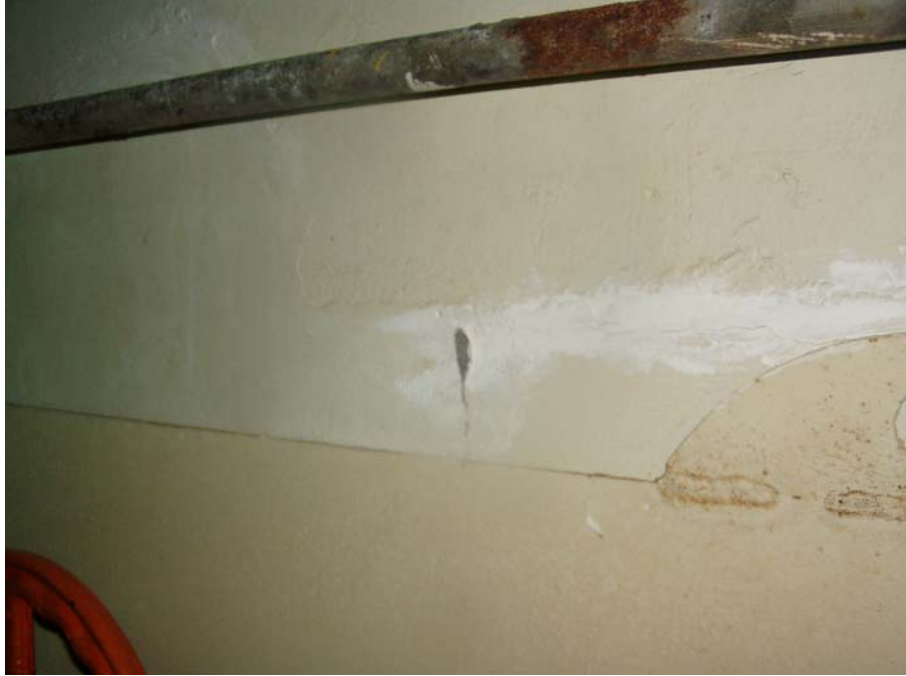
Figure 1. Entombment Top (North Side) – Surface Cracks (Typical)
