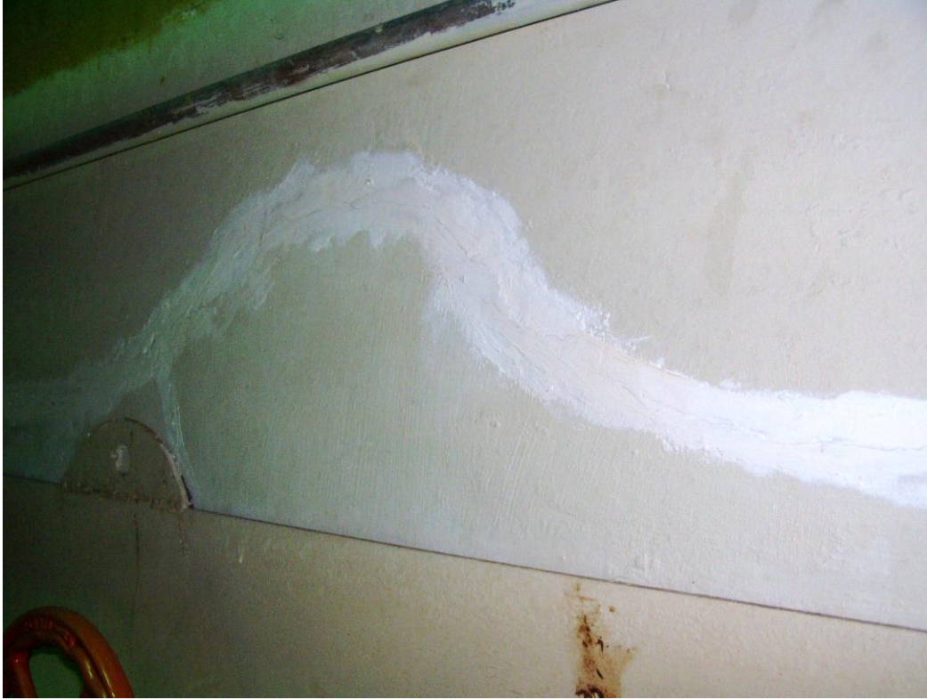
Figure 1. Entombment Top (North Side) – Surface Cracks (Typical)
