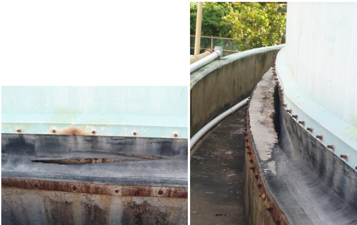
Figure 30a and 30b. Gasket Seal around Domed Metal Structure and Dome Base is Damaged and Diverts Rainwater into the Basement Level
