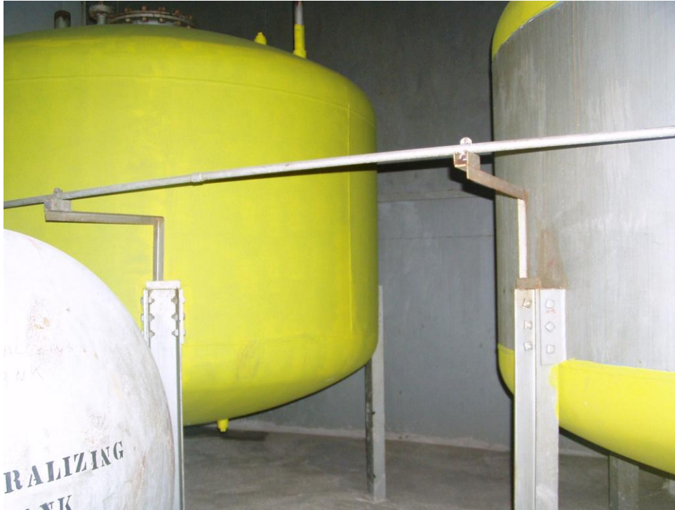
Figure 5. Basement Level – Retention Tanks 2 and 3
