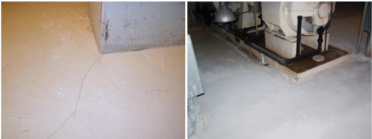
Figure 8a and 8b. Basement Level – Surface Cracks in Concrete Cover (Typical)
