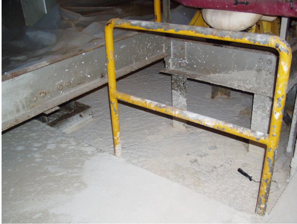
Figure 25. Basement Level – Lowest Point in Basement Shows No Recent Signs of Flooding (Dry, Cracked Silt/Mud is Visible)
