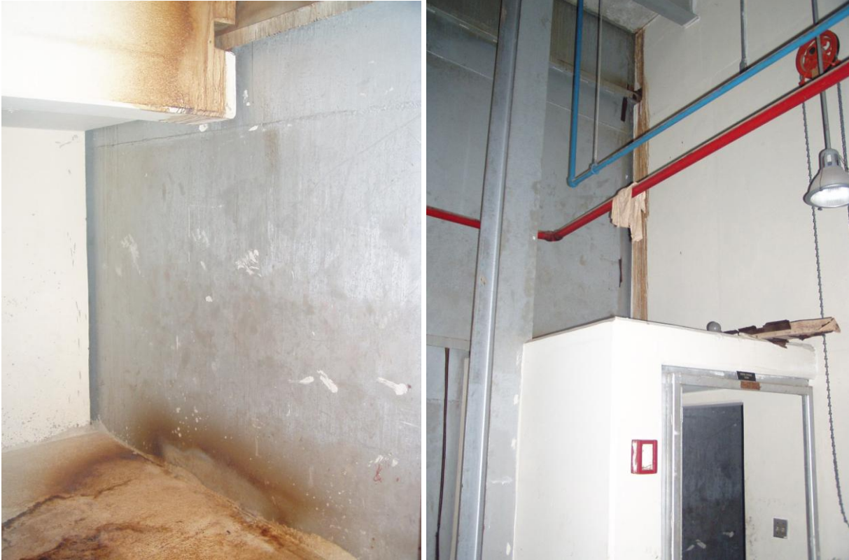
Figure 27. Basement Level – Additional View of Staining Due to Water Infiltration beneath the Northern Entrance
