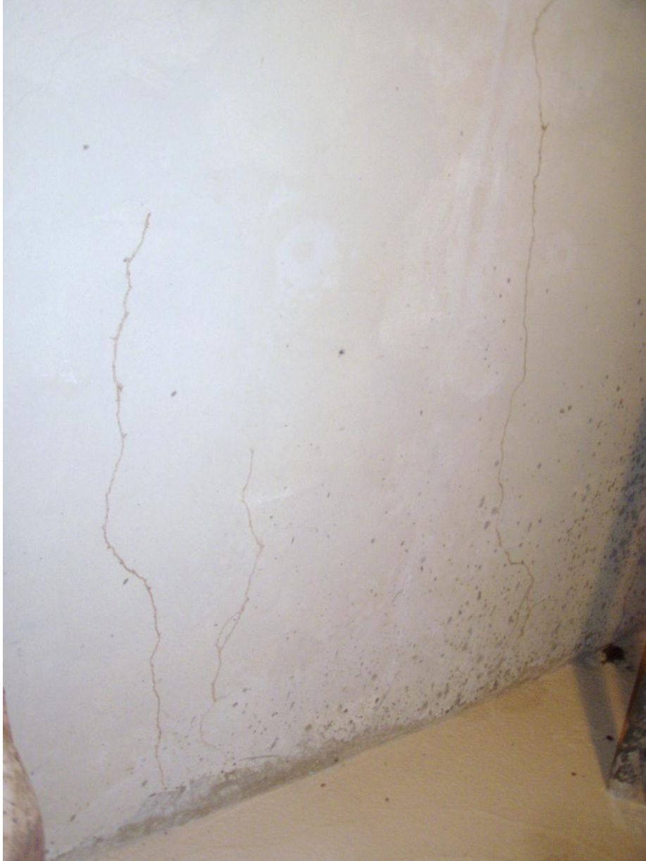
Figure 33. Basement Level – East Side Near Loading Access (Interior) with “Termite Tracks” Visible on Wall.
