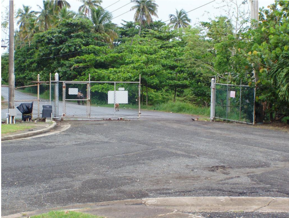
Figure 19. Site Security – Main Gate (Motor is Not Operational)
