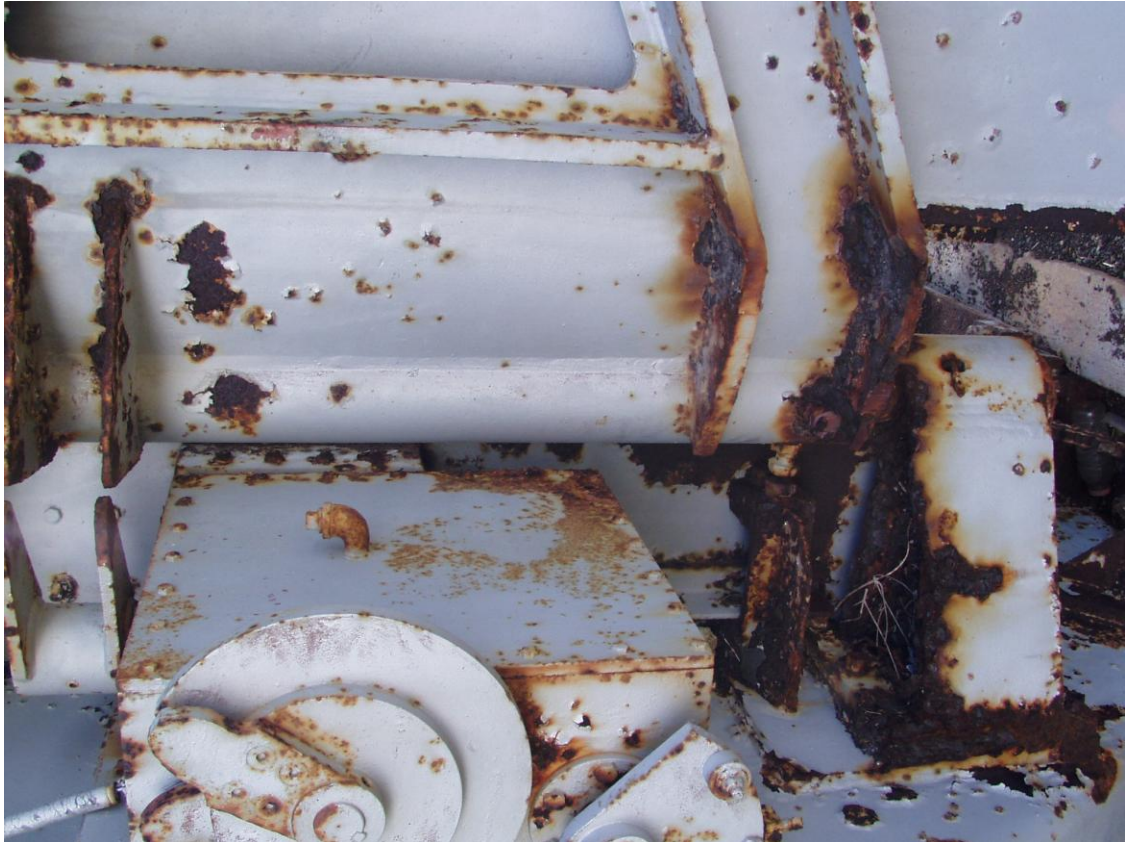
Figure 29. North Entrance – Pass-Through Chamber (Significant Corrosion)
