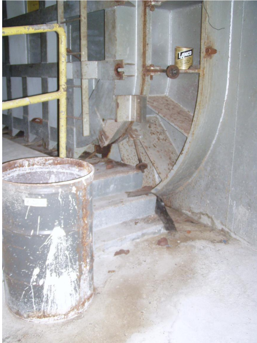
Figure 32. Basement Level – East Side Loading Access (Interior) with Water Stain Visible on Floor (Inflow through Corrosion of Metal Frame – Figure 31).
