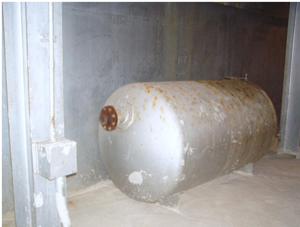
Figure 10. Basement Level – Tank Formerly Labeled as Radioactive Material/Waste Storage Tank
