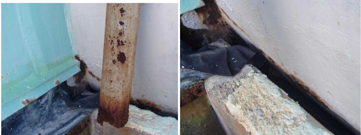
Figure 28. Gasket Seal at Northern Entrance Exterior Deteriorated
