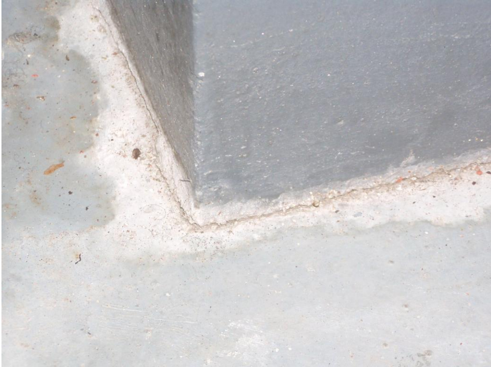
Figure 3. Entombment Top (Top Plug) – Surface Cracks (Typical)
