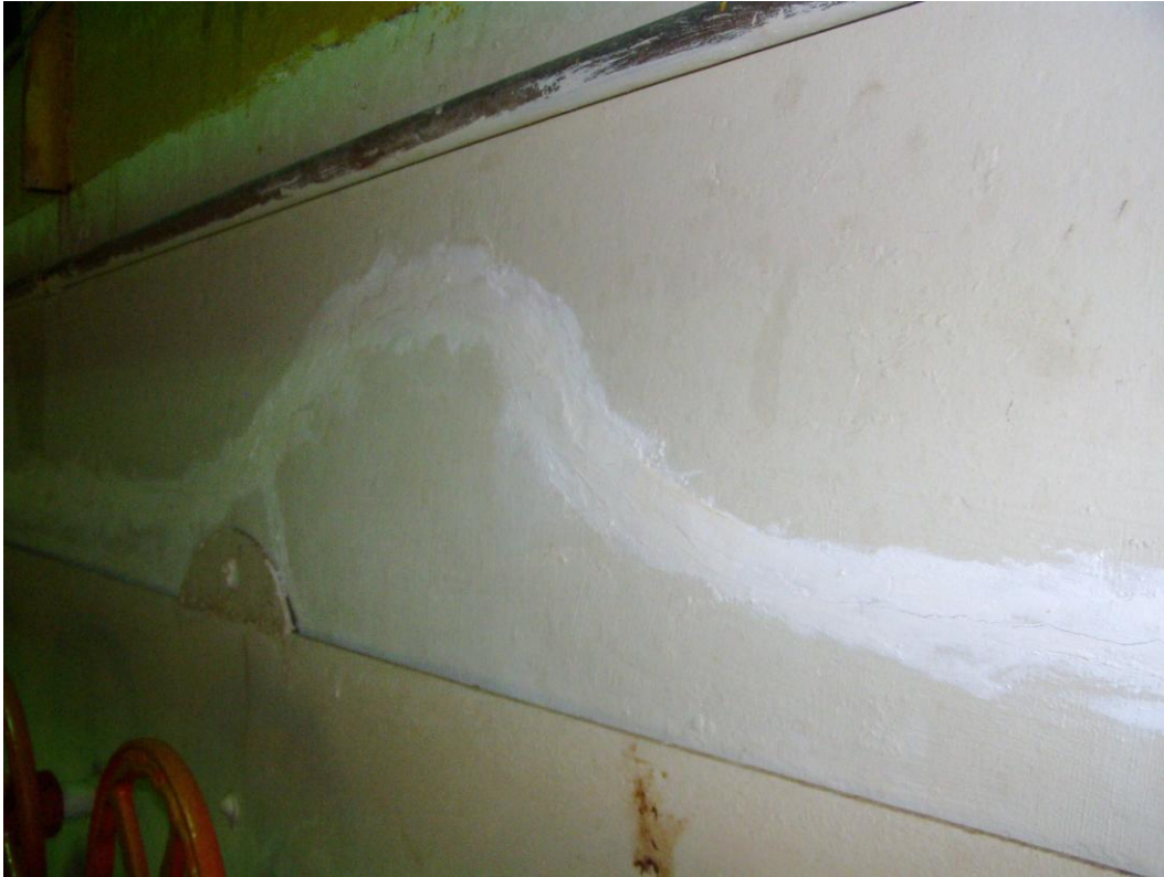
Figure 1. Entombment Top (North Side) – Surface Cracks (Typical)
