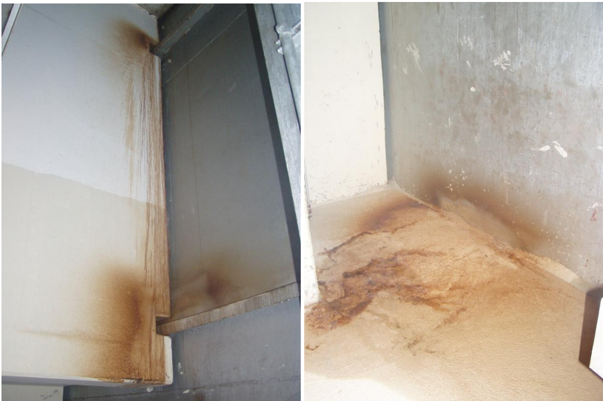
Figure 26a and 26b. Basement Level – Staining Due to Water Infiltration beneath Northern Entrance
