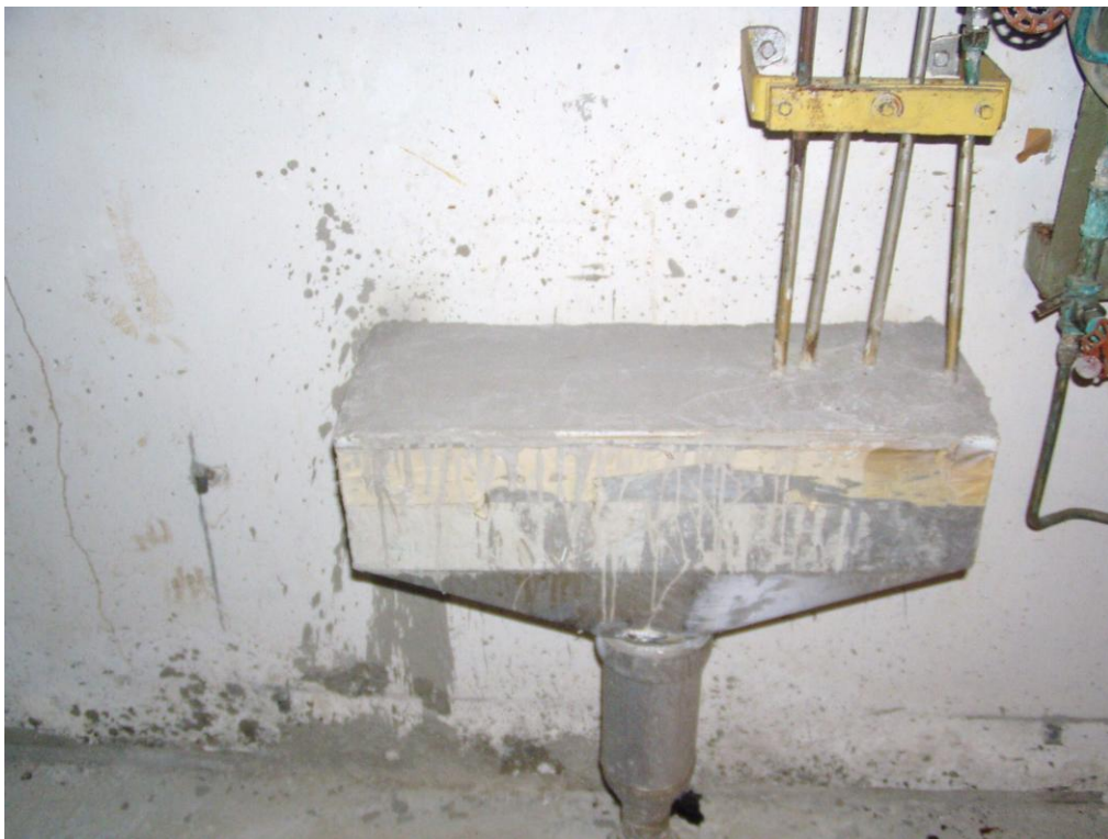
Figure 24. Basement Level – Concrete Filled Sink to Fix Removable Contamination (Good Condition)
