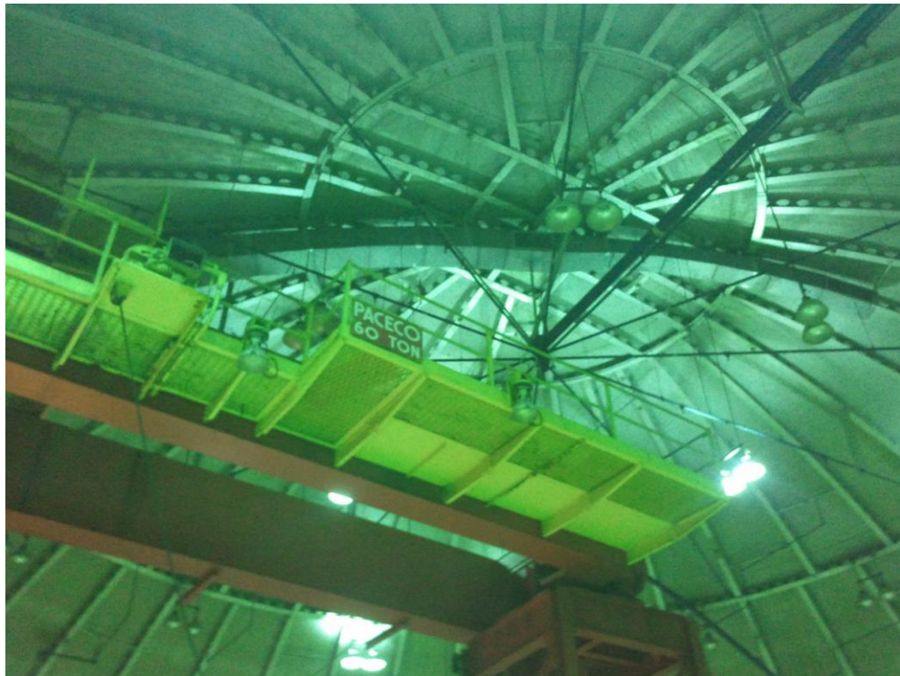
Figure 27. Dome Structure – Interior with Fire Suppression Piping
