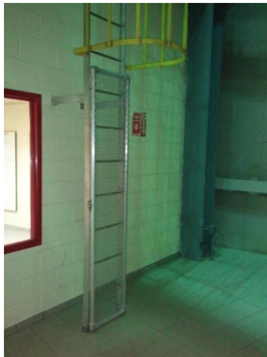
Figure 16. Main Level (Museum Area) – Ladder to Mezzanine Locked-Out
