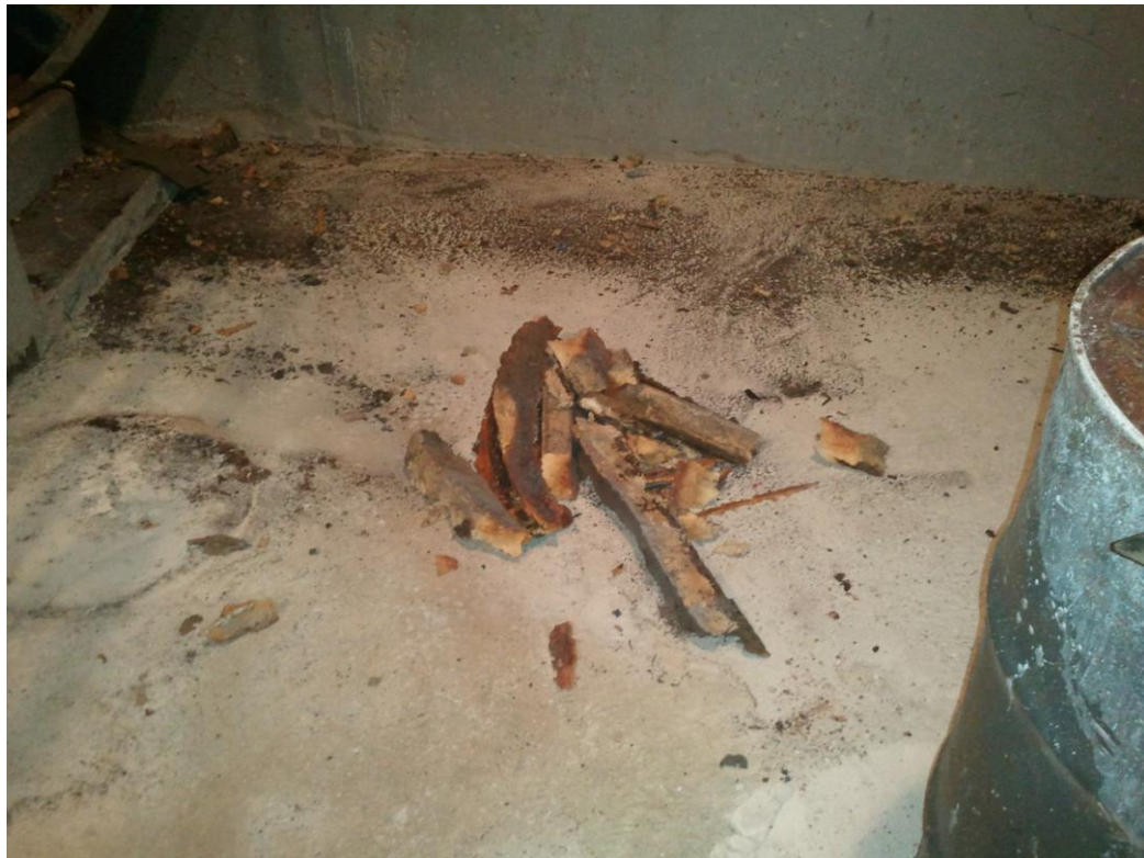
Figure 23. Basement Level – Loading Access Door (Debris from Old Seal Material)
