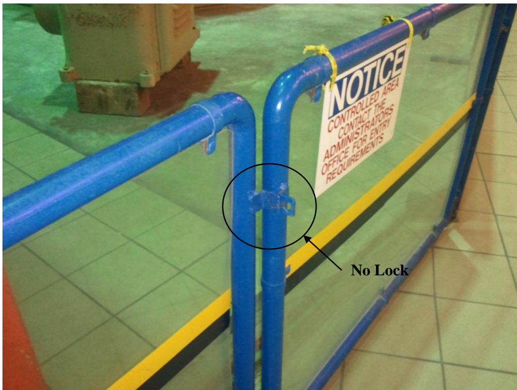
Figure 14. Main Level (Controlled Area) – Gate Access to Controlled Area
