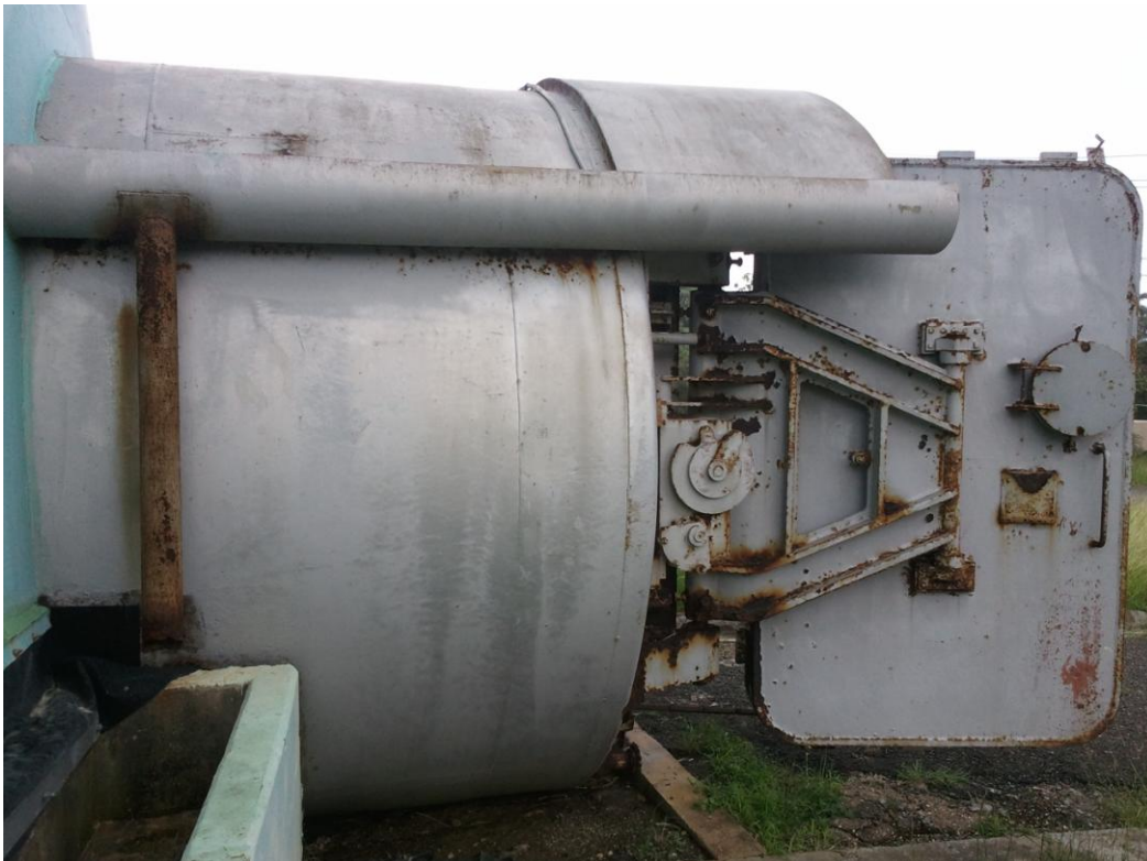
Figure 29. Dome Structure – North Entrance (Exterior with Significant Corrosion)
