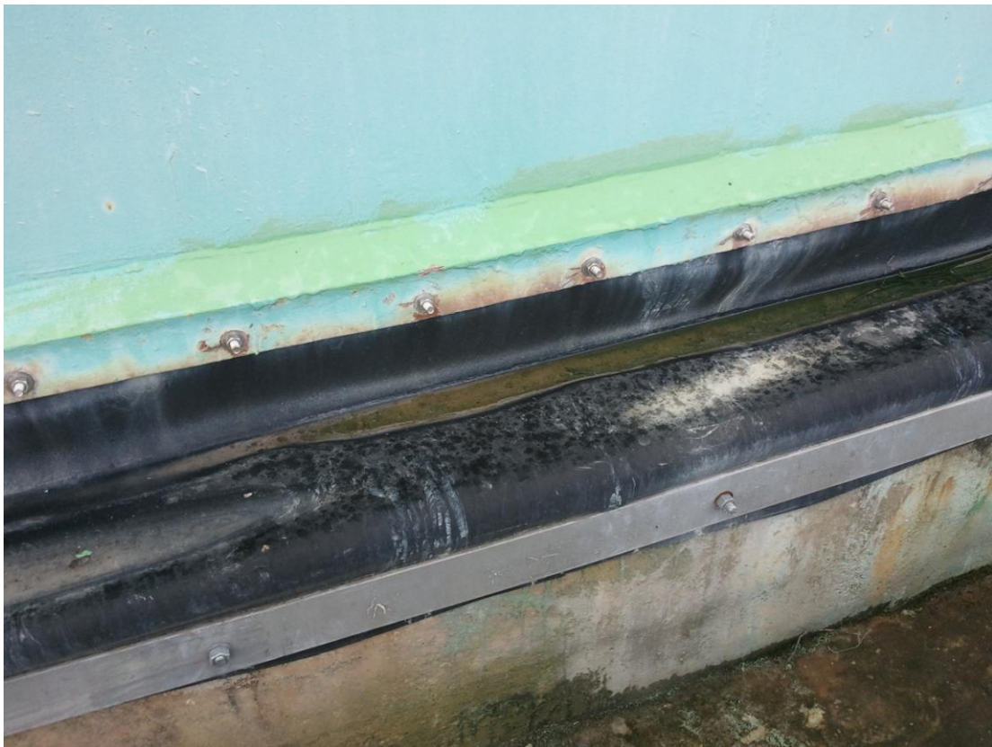
Figure 31. Dome Structure – Flexible Gasket/Seal (Retains Water in Some Locations)
