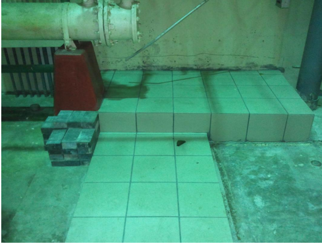
Figure 13. Main Level (Controlled Area) – Shielding with Concrete and Lead Bricks
