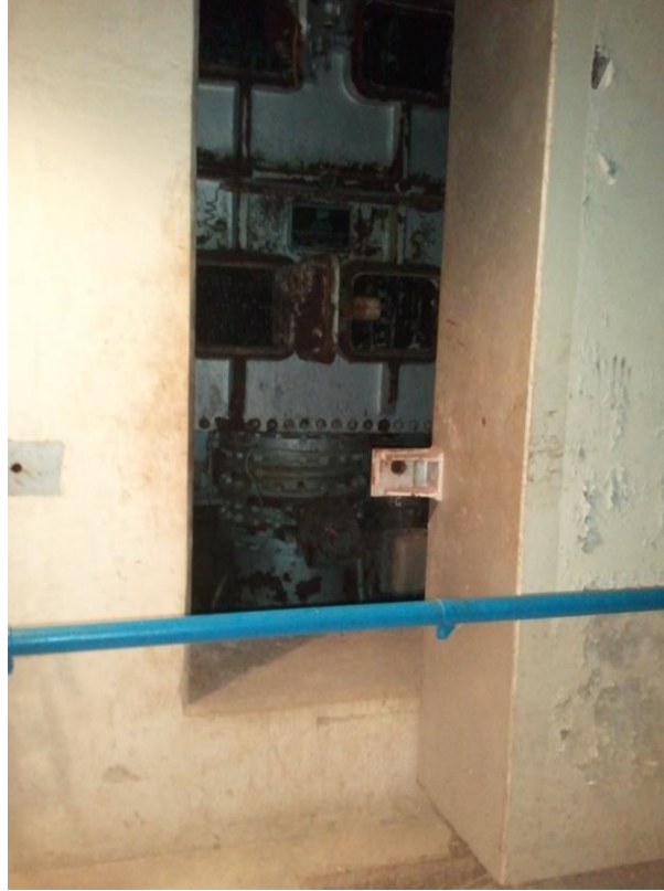
Figure 24. Basement Level – Condenser Room (North Side Access)
