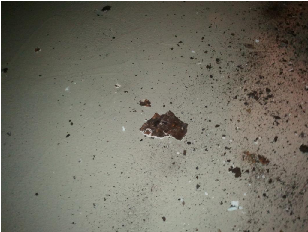
Figure 25. Basement Level – Condenser Room (Debris from Condenser on Floor)
