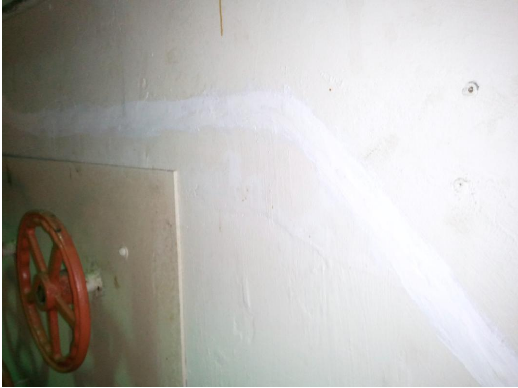
Figure 1. Entombment Top (North Side) – Surface Cracks (Typical)
