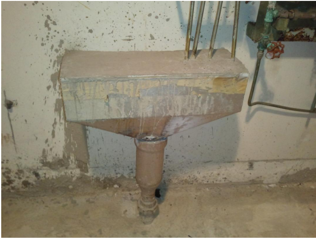
Figure 19. Basement Level – Concrete Filled Sink
