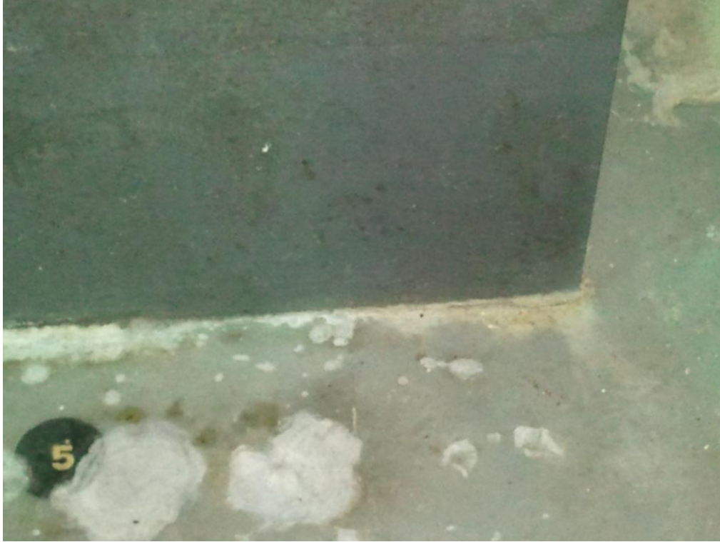
Figure 3. Entombment Top (Top Plug) – Surface Cracks (Typical)
