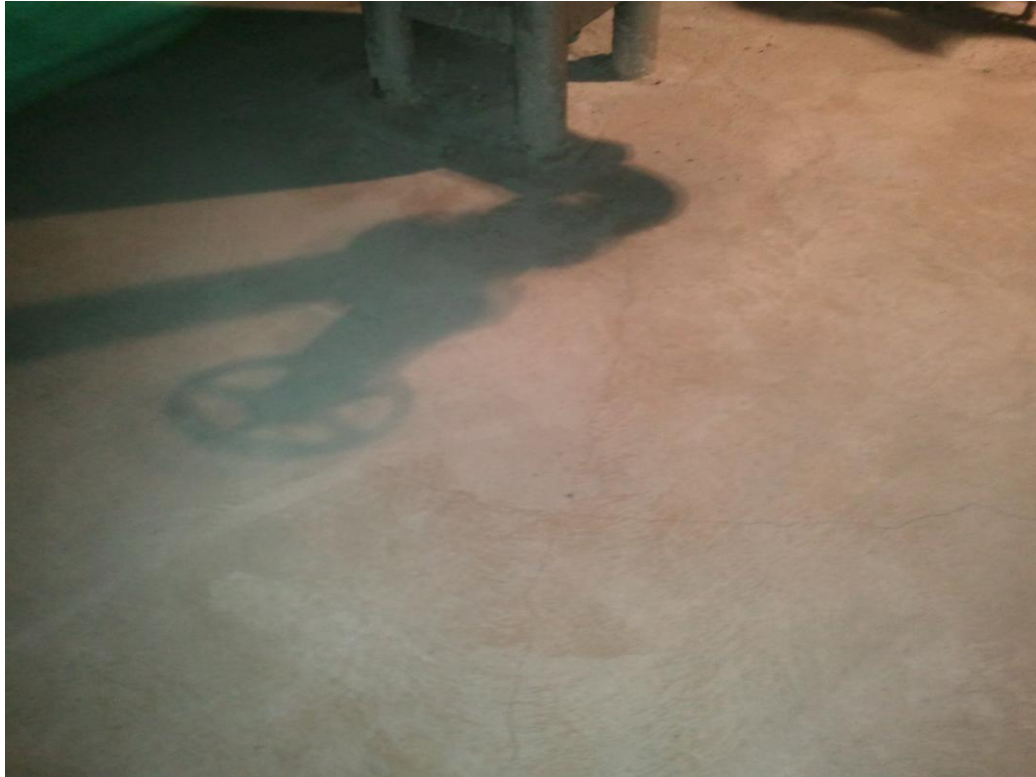
Figure 17. Basement Level – Cracks in Concrete Floor (Typical)
