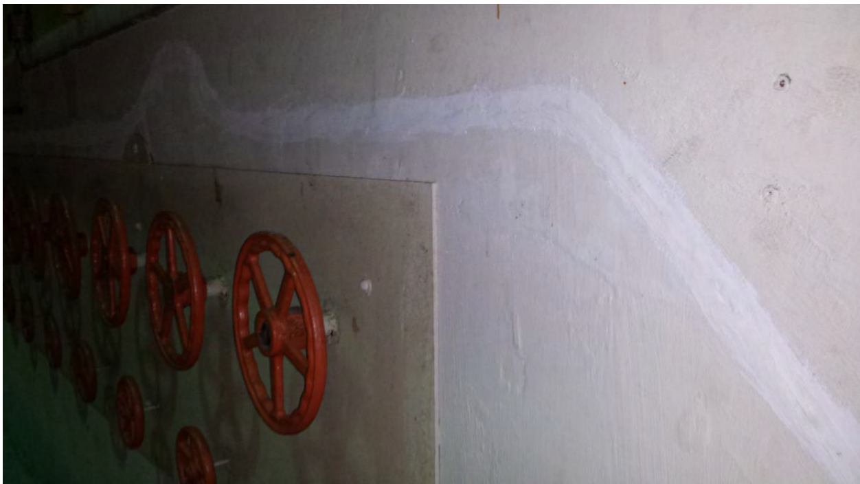
Figure 4. Entombment Top – Surficial Cracks (Typical)
