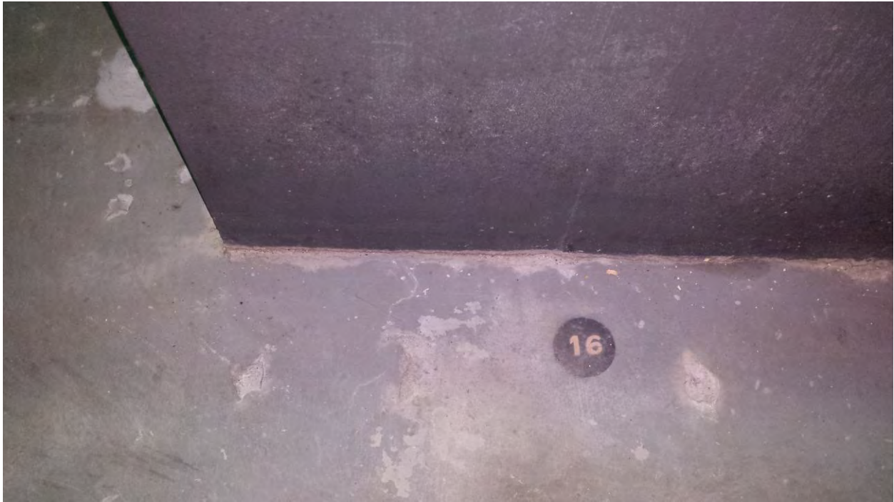
Figure 1. Entombment Top (Top Plug, South Side) – Sampling Point 16 and Surface Cracks (Typical)
