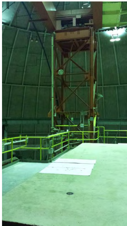
Figure 2. Entombment Top (Crane) – Absorbent Pads Placed to Contain Oil/Lubricant Drips from Overhead Crane Equipment
