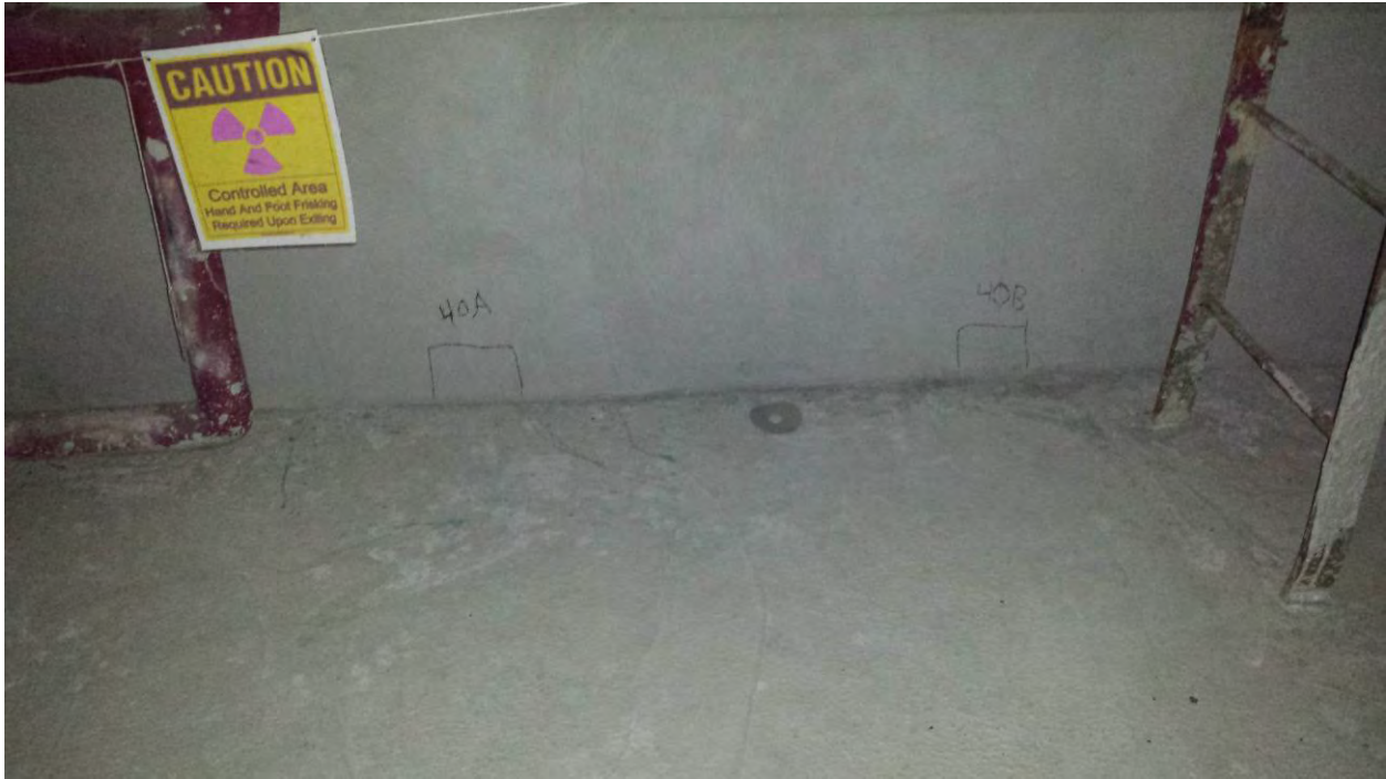
Figure 19. Basement Level – Sample Locations 40A and 40B Covered by Engineering Control (~1/2 Inch Concrete) with Caution Sign Reading “Controlled Area – Hand and Foot Frisking Required Upon Exit”
