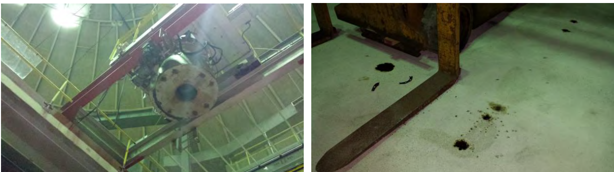
Figure 29. Basement Level – Oil Leaking on Basement Floor from Overhead Machinery
