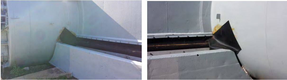
Figure 27. Dome Structure – Flexible Gasket/Seal – North Entrance Air Lock (Several Repairs have been Made)
