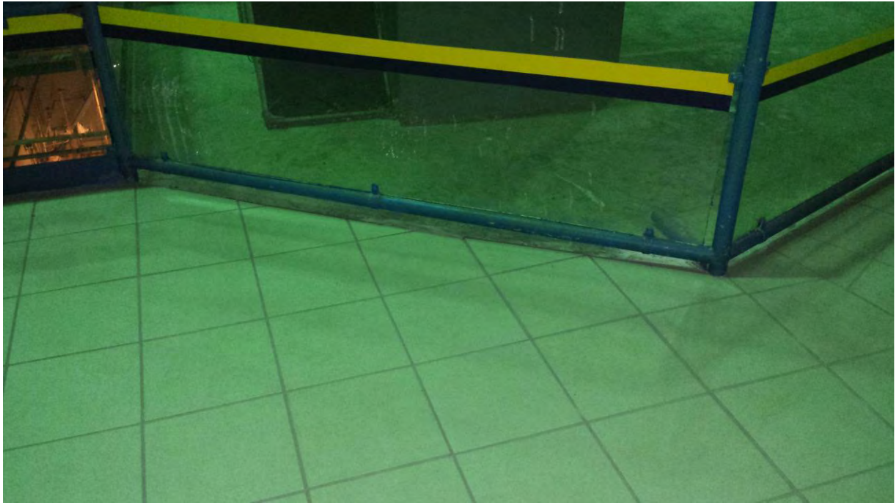
Figure 30. Main Level (Museum Area) – Some Tiles Starting to Loosen
