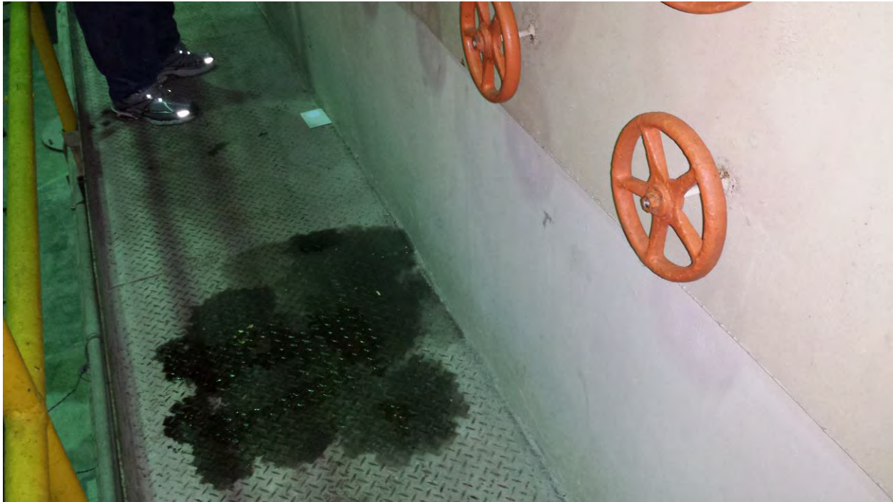
Figure 3. Entombment Top – Oil Leaking from Overhead Crane (Near Sampling Points 1, 2, 3, and 4)
