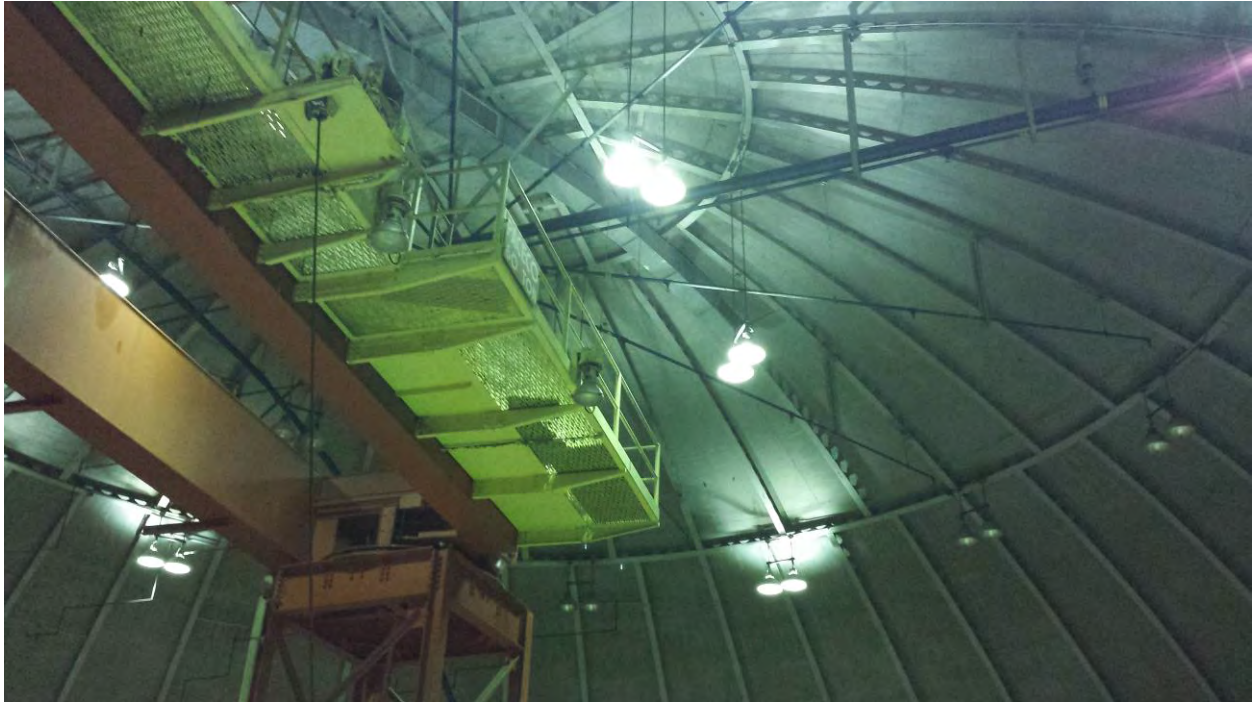
Figure 24. Dome Structure – Interior with Fire Suppression Piping
