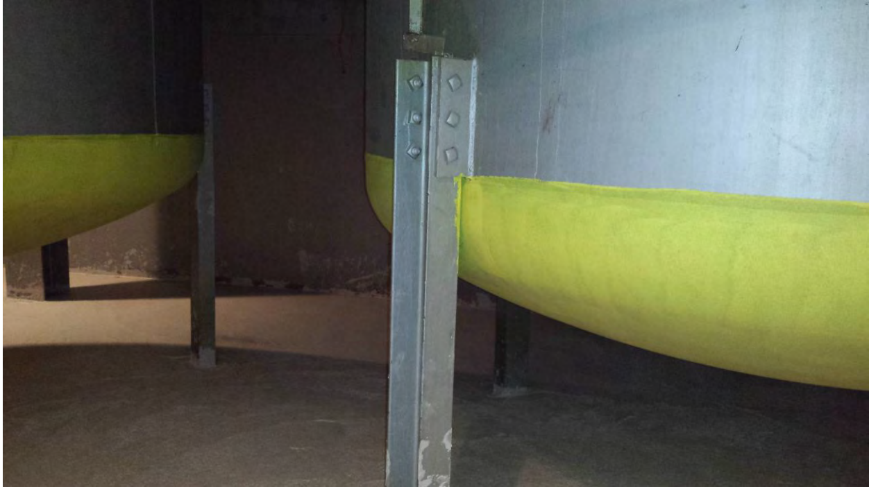
Figure 21. Basement Level – Liquid Water Retention Tanks #1, #2, and #3 with Engineering Control (Yellow Paint) Starting to Show Signs of Thinning
