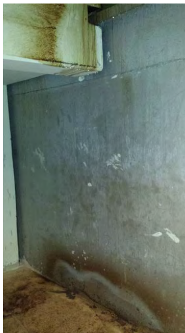
Figure 16. Basement Level – Beneath North Entrance Air Lock (No Signs of Recent Water Infiltration – Older Stains Persist)
