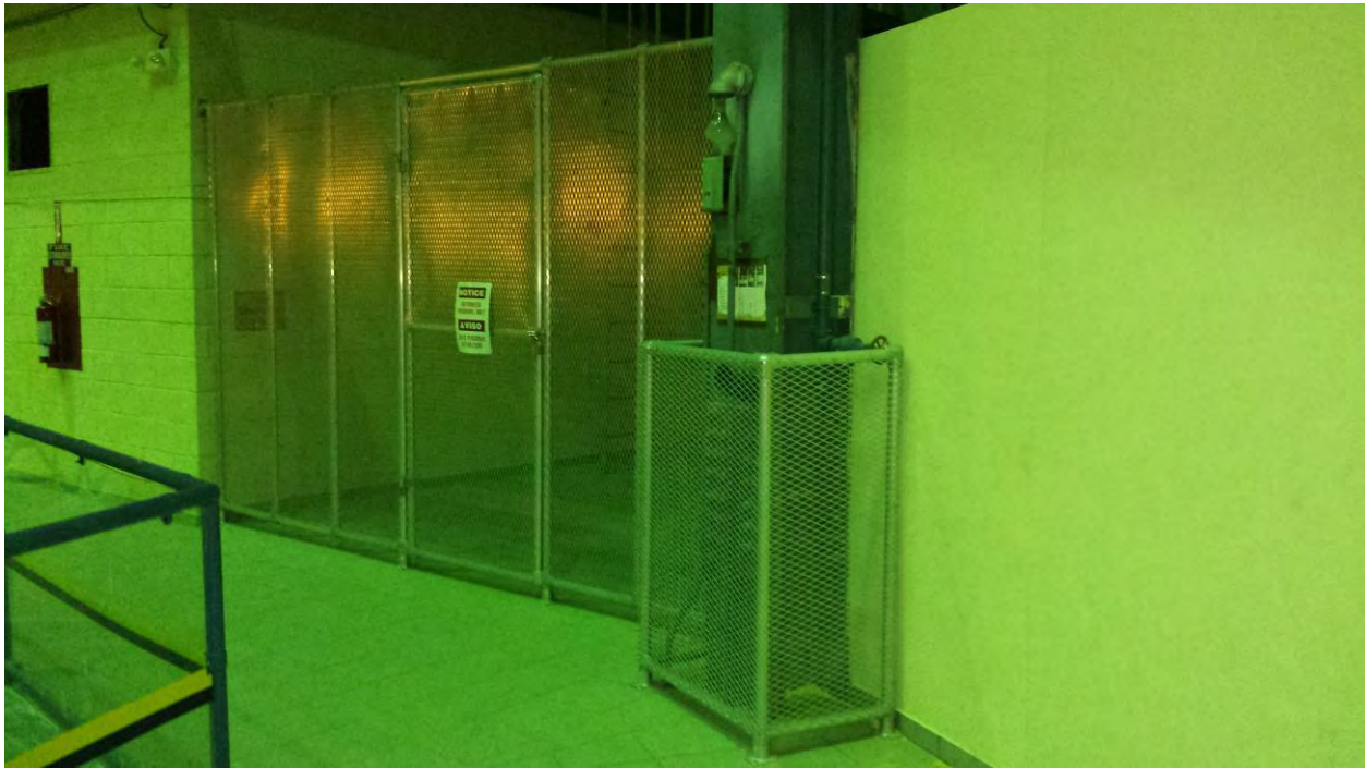
Figure 11. Main Level – Locked and Controlled Access to East Mezzanine and Electrical Panels
