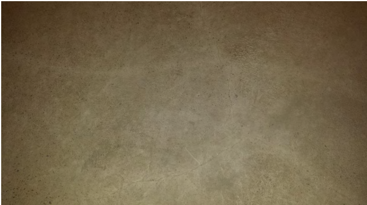
Figure 20. Basement Level – Engineering Control (~6 Inch Concrete Floor Covering) with Surficial Cracks (Typical)
