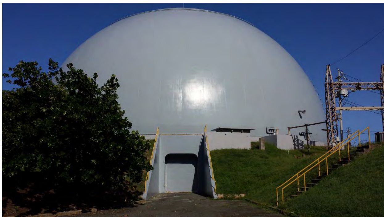
Figure 15. Basement Level (Exterior) – Bay Door Sealed with Expanding Foam to Prevent Rain Water Infiltration
