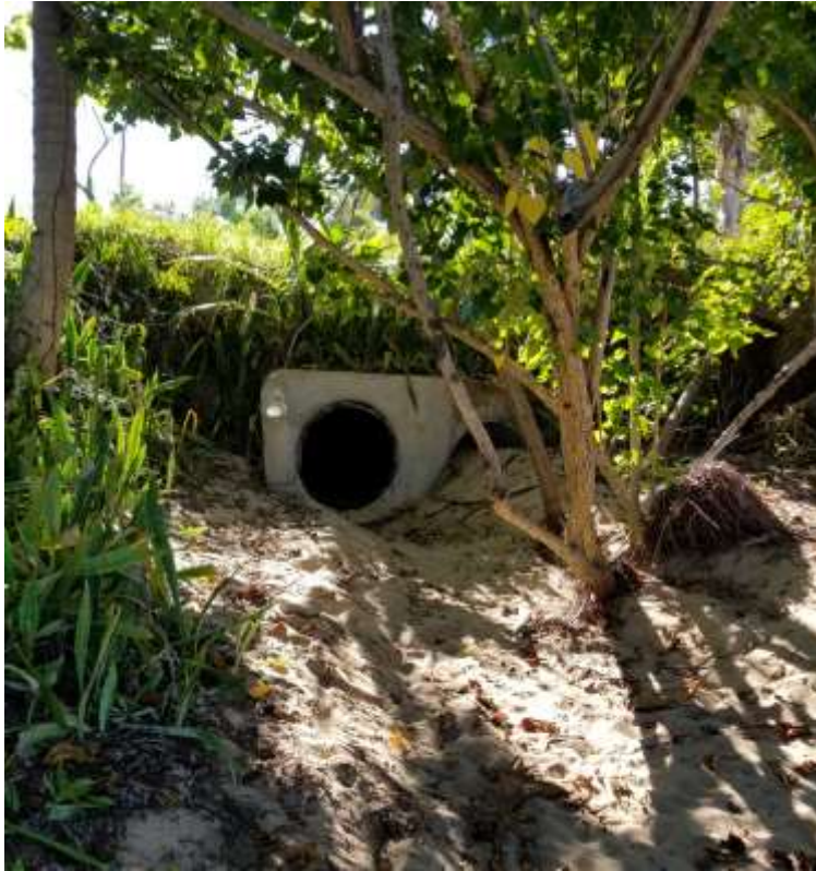
Debris Blocking Pipes on East Side of Road
