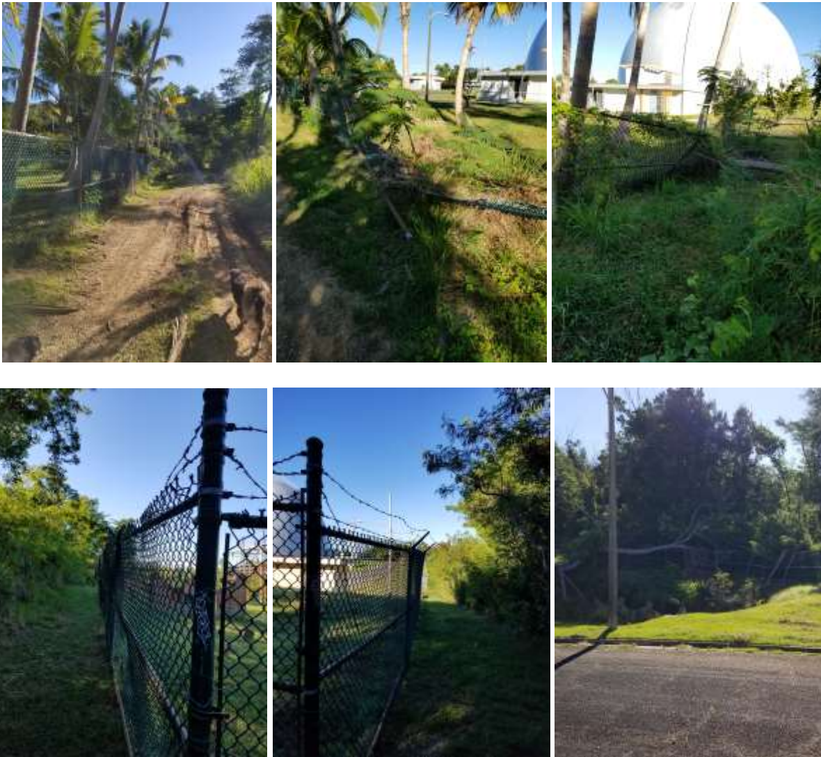
Figure 36. Fence –Fencing and Perimeter – 2017 Hurricane Season Damaged Several Sections of Fencing (Approximately 100-ft Total Length)
