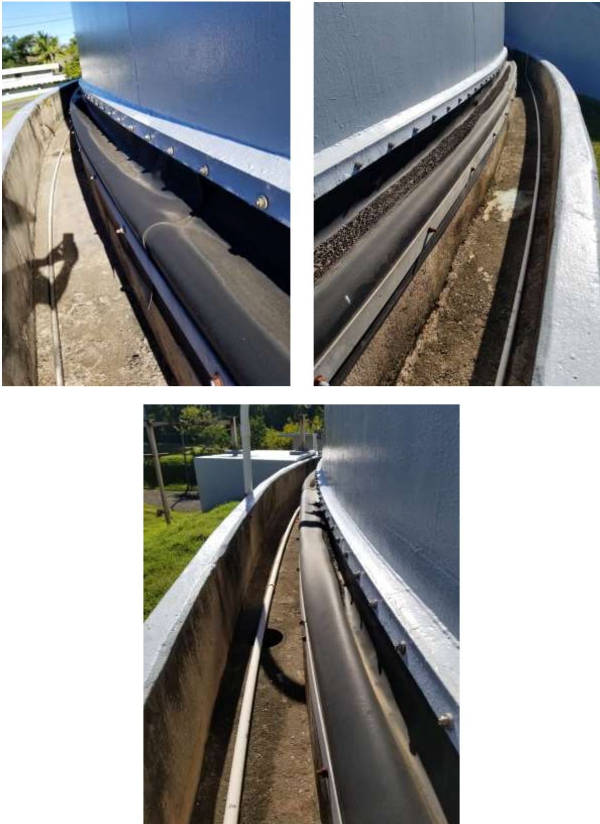
Figure 38. Dome Structure – Rain Trough Below Flexible Gasket/Seal (Drain is Free of Debris)
