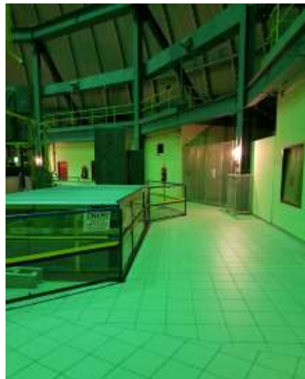
Figure 11. Main Level – Locked and Controlled Access to East Mezzanine and Electrical Panels
