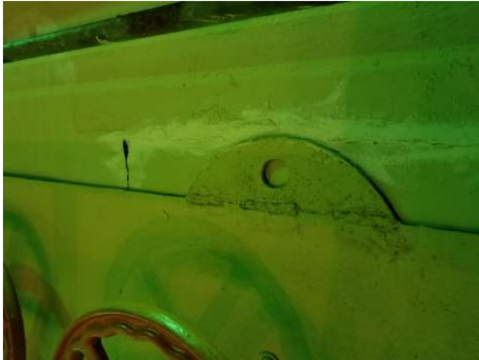
Figure 3. Entombment Top – Surficial Cracks (Typical)
