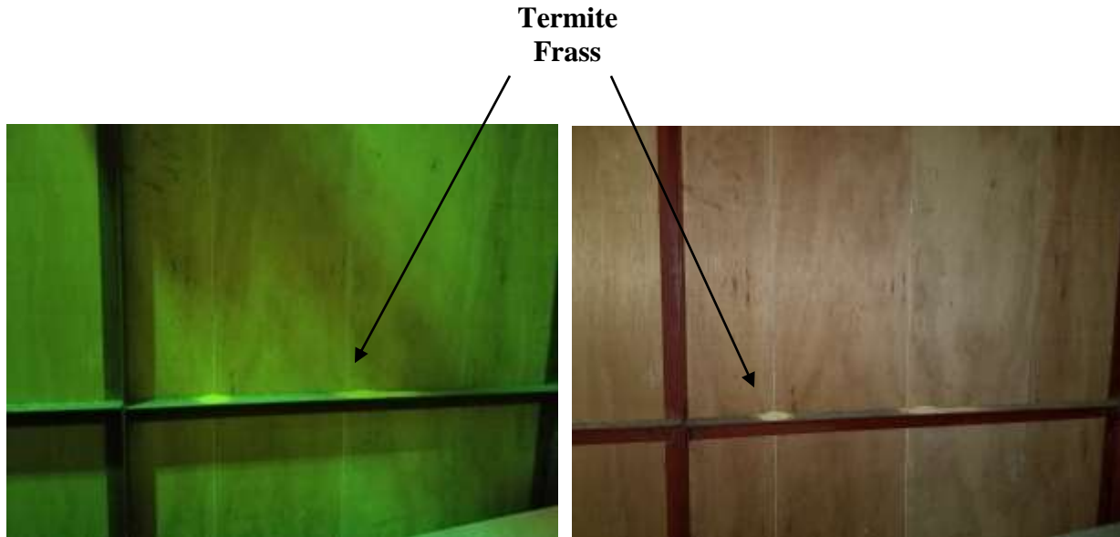
Figure 22. Main Level (Museum Area) – Wood Paneling with Past Evidence of Termites (East Side)
