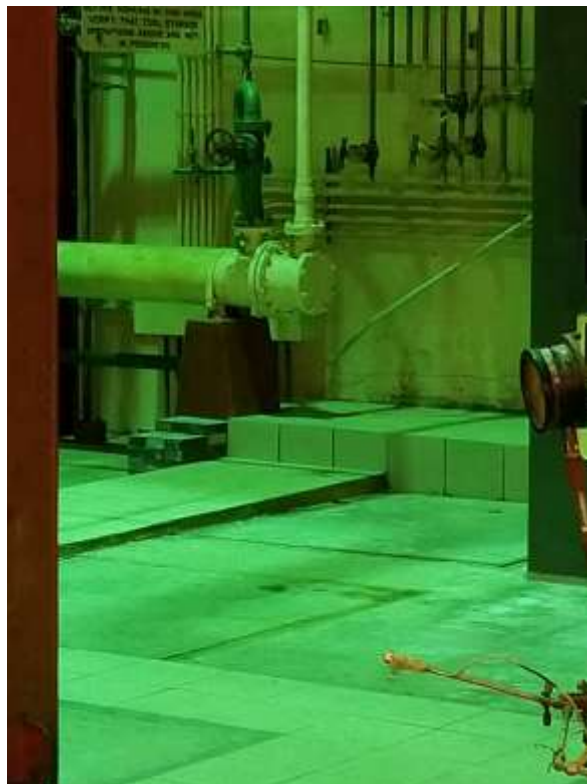
Figure 21. Main Level (Controlled Area) – Engineering Controls (Concrete, Tiles, and Lead Bricks) in Good Condition
