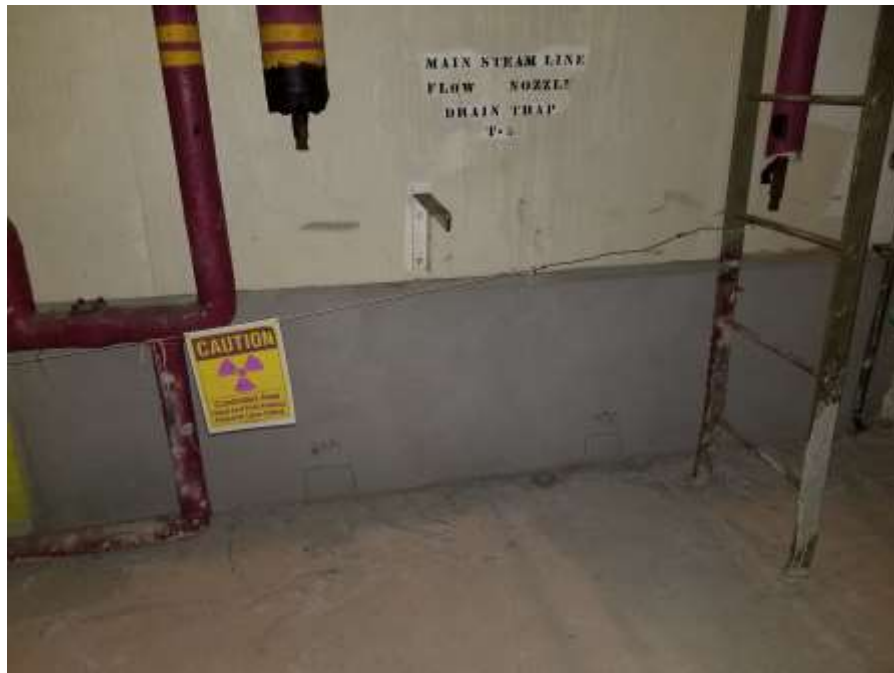
Figure 28. Basement Level – Sample Locations 40A and 40B Covered by Engineering Control (~1/2 Inch Concrete) with Caution Sign Reading “Controlled Area – Hand and Foot Frisking Required Upon Exit”
