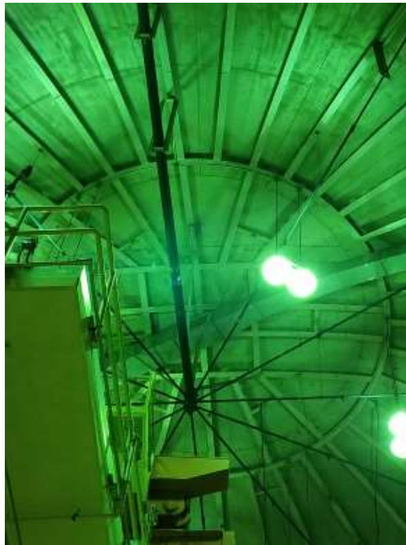
Figure 33. Dome Structure – Interior with Fire Suppression Piping
