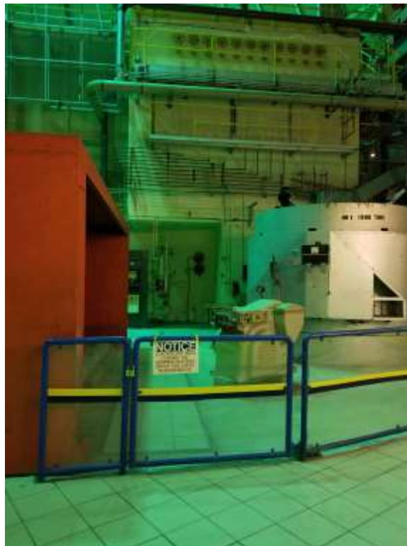
Figure 15. Main Level (Controlled Area) – Locked Access from Museum Area to Controlled Area
