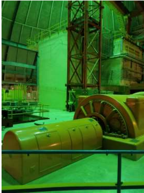
Figure 18. Main Level (Controlled Area) –Northeast Side
