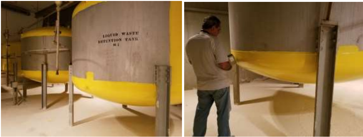
Figure 30. Basement Level – Sample Locations #30 and #31 on Liquid Waste Retention Tanks with Engineering Control (Yellow Paint) – Showing Signs of Wear
