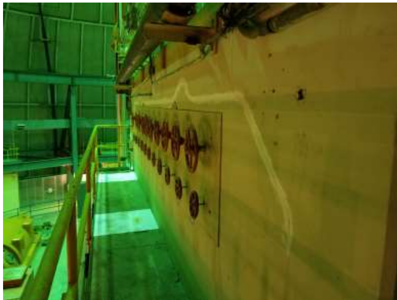
Figure 2. Entombment Top – Pad has been Placed to Address Oil Leaking from Overhead Crane (Near Sampling Points 1, 2, 3, and 4)
