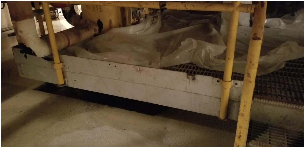
Figure 27. Basement Level – Lowest Point in Basement with No Standing Water in Sump (1- to 2-Inches of Water on Floor Due to Accidental Flooding)
