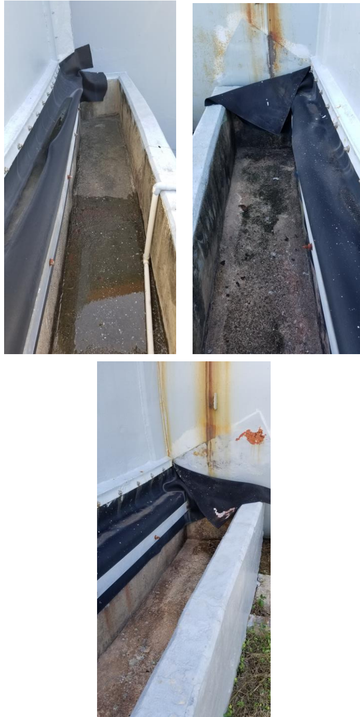
Figure 38. Dome Structure – Rain Trough Below Flexible Gasket/Seal (Drain is Free of Debris)
