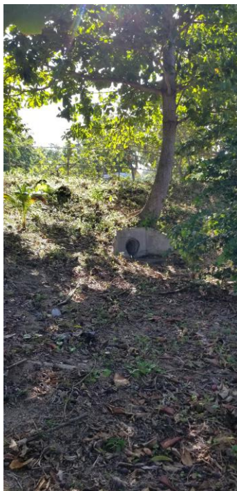
Figure 34. Dome Structure – Drainage Outfall Points and Ditches (Southern Outfall)
