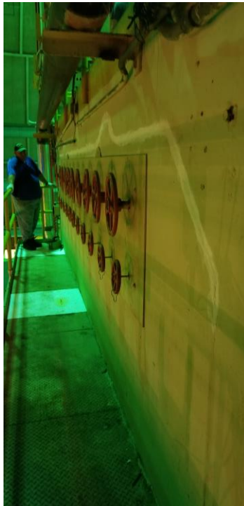
Figure 2. Entombment Top – Pad has been Placed to Address Oil Leaking from Overhead Crane (Near Sampling Points 1, 2, 3, and 4)
