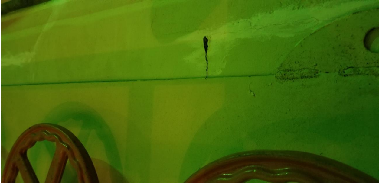
Figure 3. Entombment Top – Surficial Cracks (Typical)
