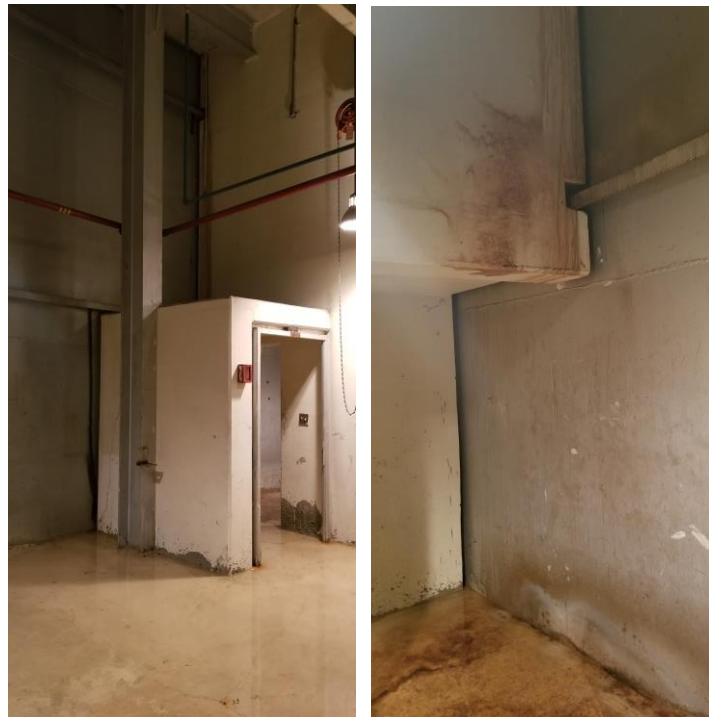
Figure 25. Basement Level – Beneath North Entrance Air Lock (No Signs of Recent Water Infiltration – Older Stains Persist) – 1- to 2-Inches of Water on Floor Due to Accidental Flooding
