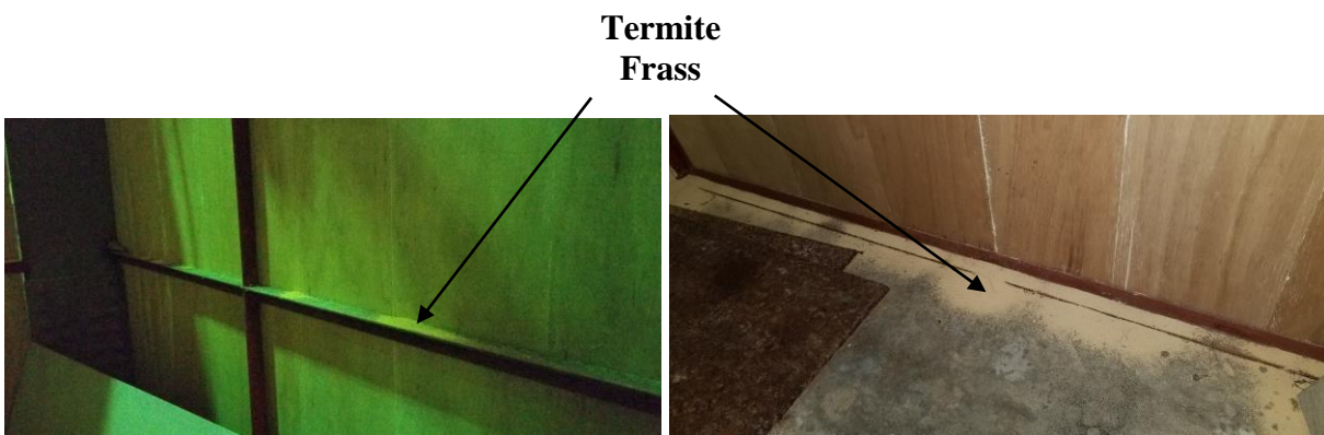
Figure 22. Main Level (Museum Area) – Wood Paneling with Past Evidence of Termites (East Side)
