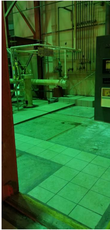
Figure 21. Main Level (Controlled Area) – Engineering Controls (Concrete, Tiles, and Lead Bricks) in Good Condition
