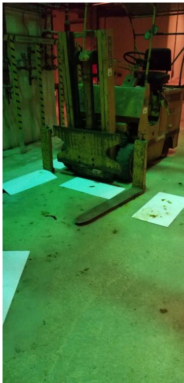
Figure 24. Basement Level – Oil/Lubricant Spots on Basement Floor from Overhead Equipment (1- to 2-Inches of Water on Floor)
