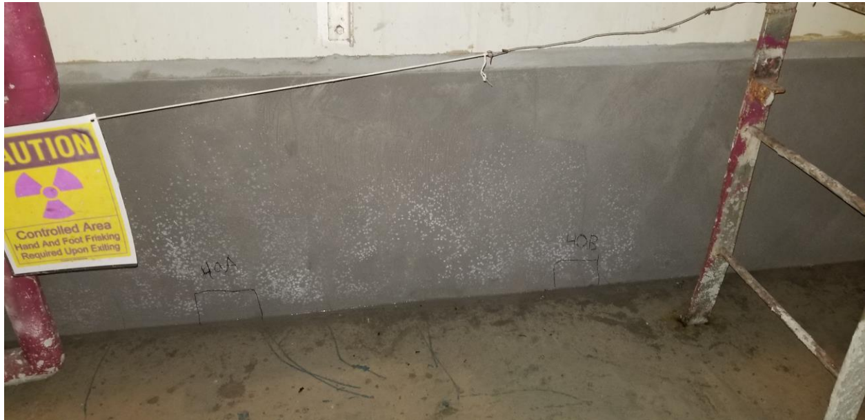
Figure 28. Basement Level – Sample Locations 40A and 40B Covered by Engineering Control (~1/2 Inch Concrete) with Caution Sign Reading “Controlled Area – Hand and Foot Frisking Required Upon Exit” (Water on Floor)
