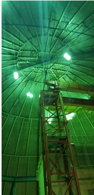
Figure 33. Dome Structure – Interior with Fire Suppression Piping
