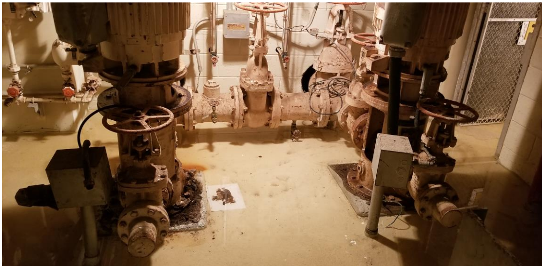
Figure 31. Basement Level – Condensate Pumps #1 and #2 with Loose/Removable Contaminated debris (1- to 2-Inches of Water on Floor)
