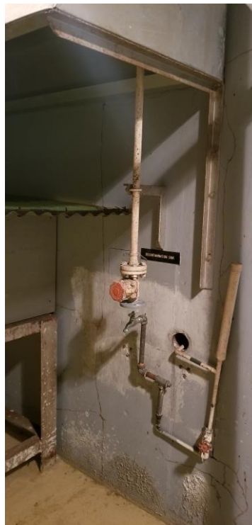
Figure 29. Basement Level – Painted Flange (Engineering Controls) at Former Decontamination Sink Location
