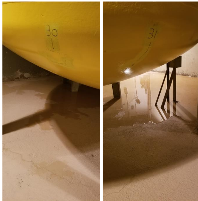
Figure 30. Basement Level – Sample Locations #30 and #31 on Liquid Water Retention Tanks with Engineering Control (Yellow Paint) – Showing Signs of Wear
