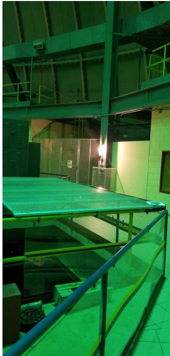
Figure 11. Main Level – Locked and Controlled Access to East Mezzanine and Electrical Panels
