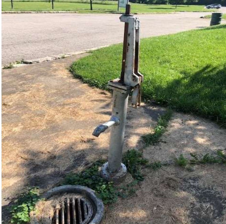
P15 – Handpump Well (#5160) at Red Gate Woods Parking Lot
