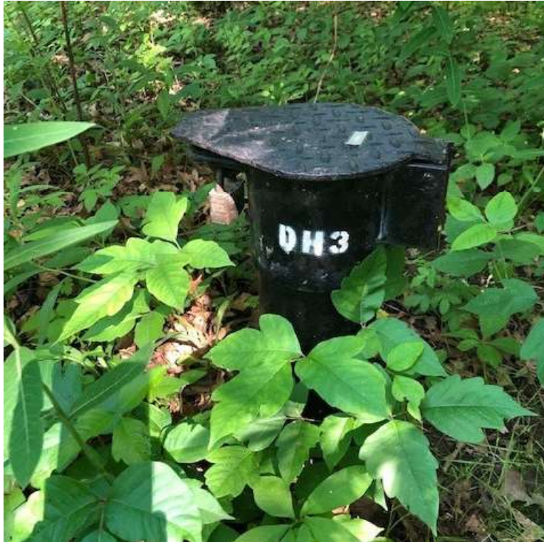
P11 – Monitoring Well DH3 at Red Gate Woods
