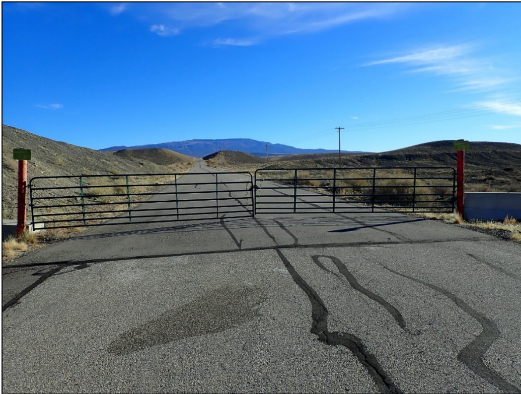
PL-1. Site Access Gate
