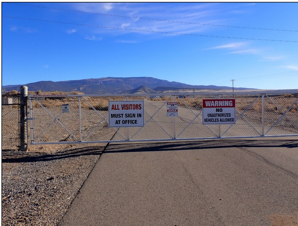
PL-3. Solar-Powered Site Entrance Gate
