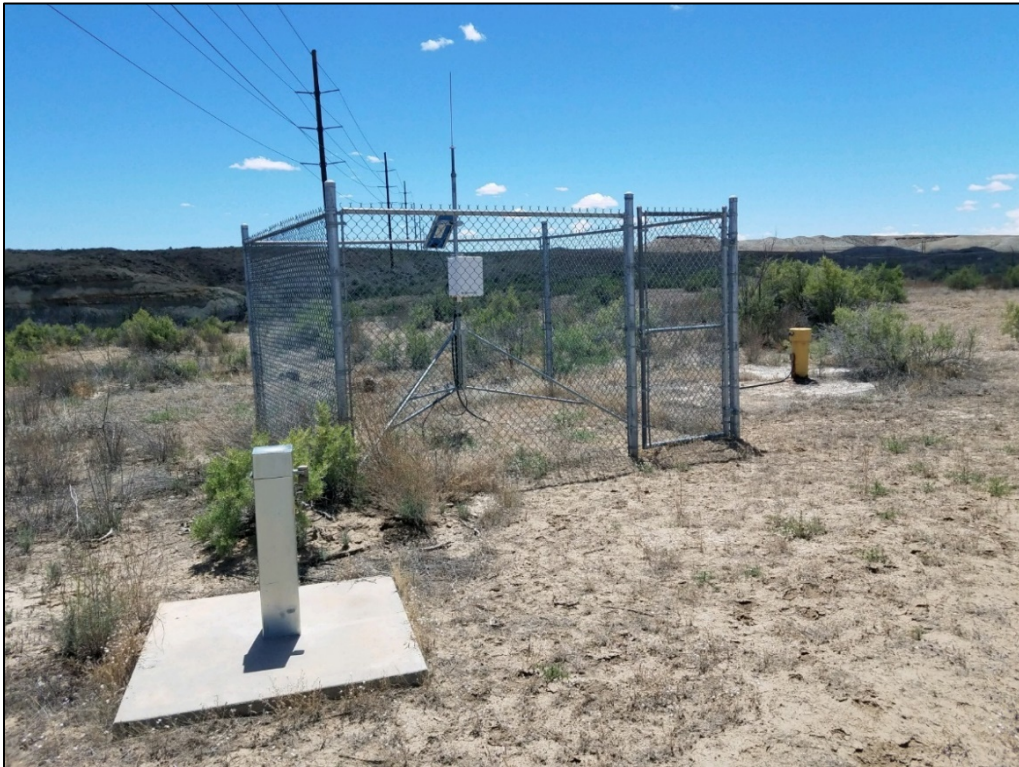
PL-6. Monitoring Wells 0194 and 0582 (with the System Operation and Analysis at Remote Sites [SOARS] Station in Background)
