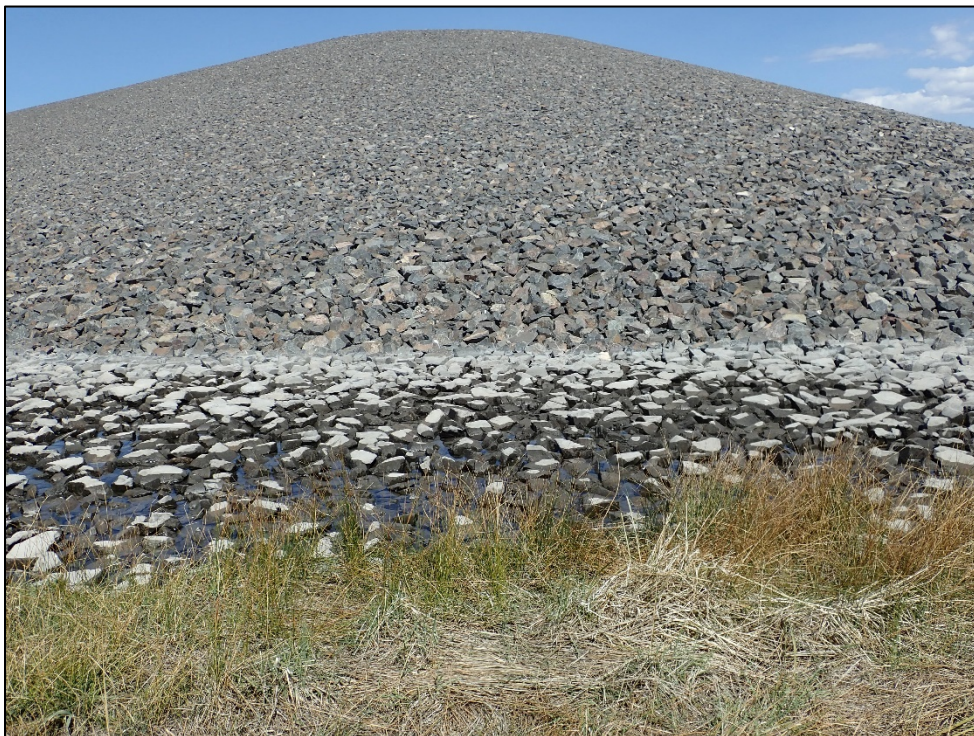
PL-6. Water in Cell Apron, Southeast Corner
