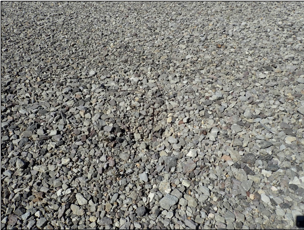
PL-10. Shallow Depression No. 3 on Disposal Cell Top Slope
