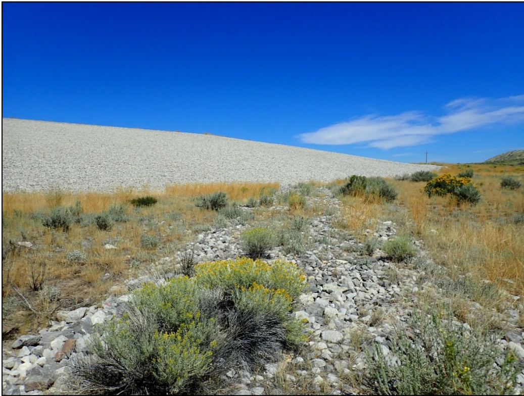
PL-14. Apron Toe Drain North of Ancillary Cell and Disposal Cell South Side Slope in Background
