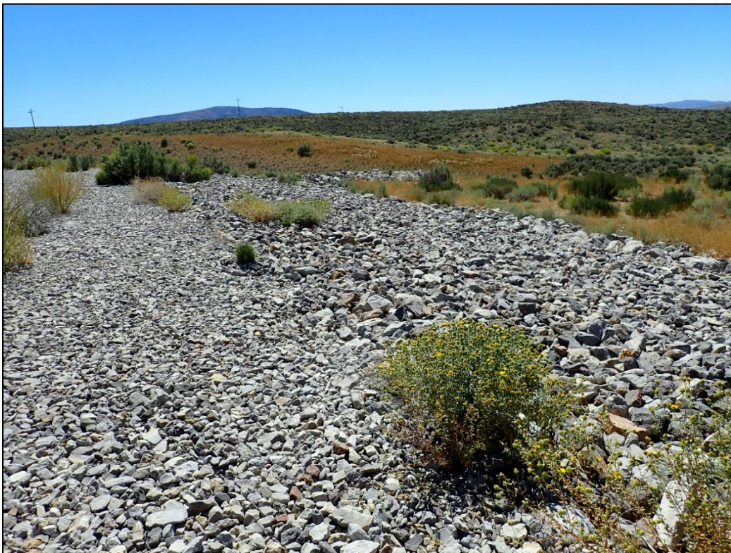
PL-16. Ancillary Cell West Side Slope with Small Depression on Cell Top Slope in Foreground
