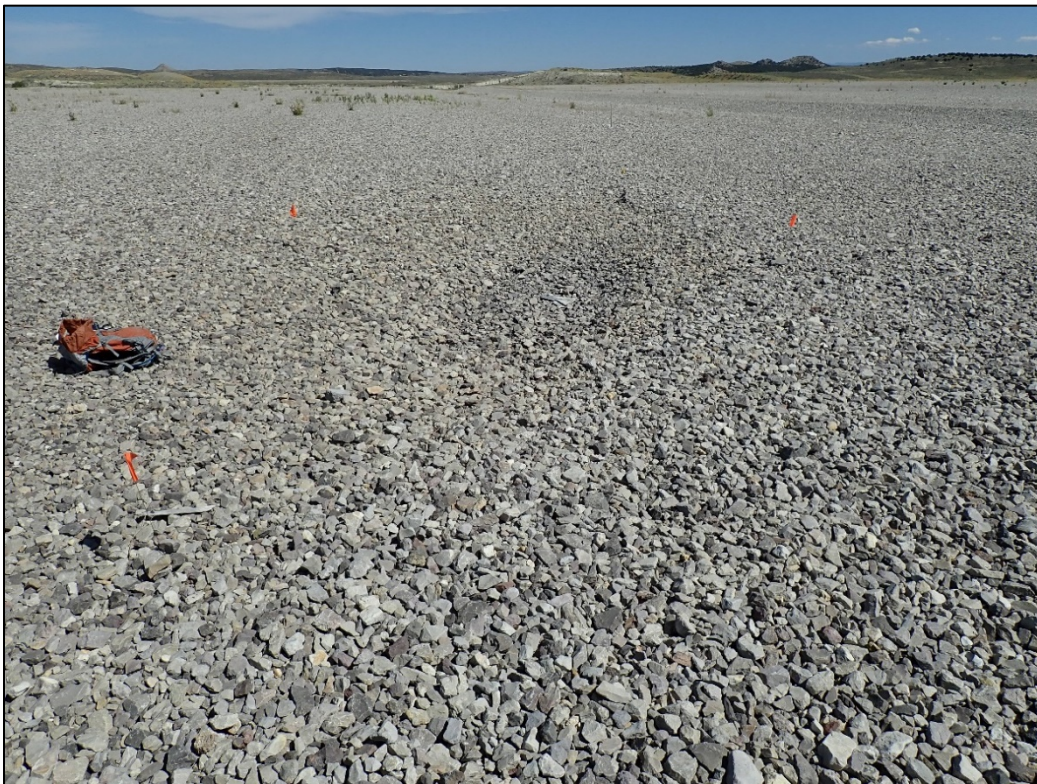
PL-8. Shallow Depression No. 1 on Disposal Cell Top Slope
