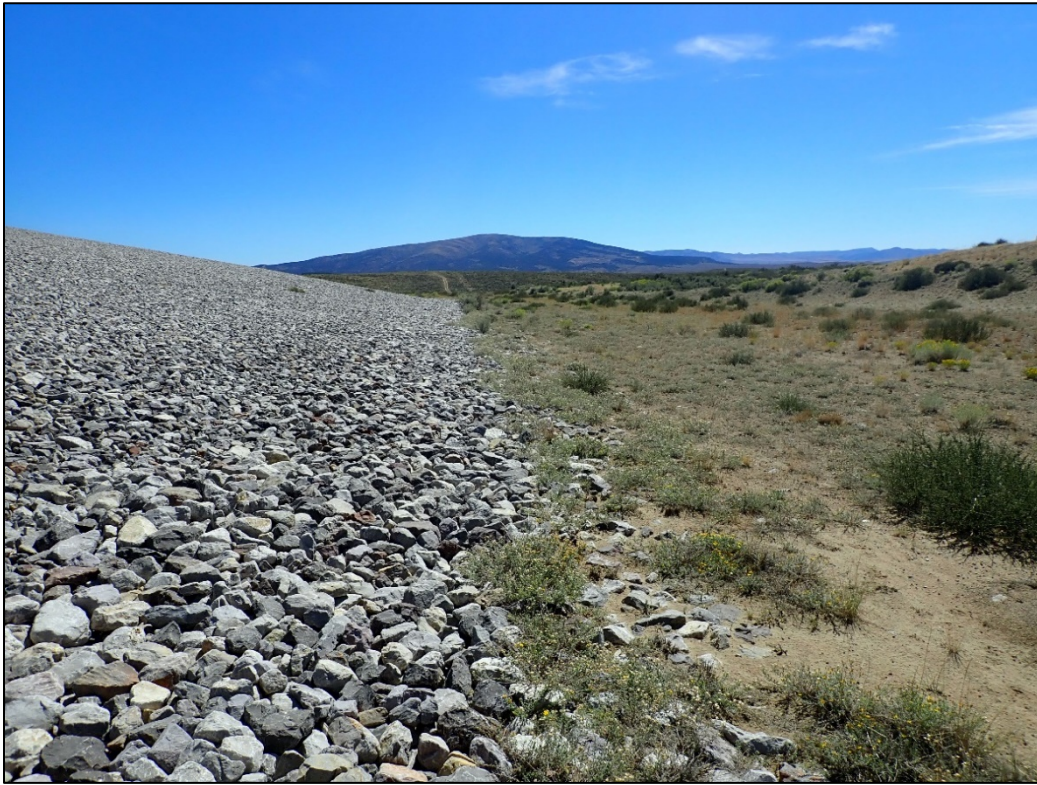
PL-13. Windblown Sediment Accumulating at Toe of Disposal Cell West Side Slope
