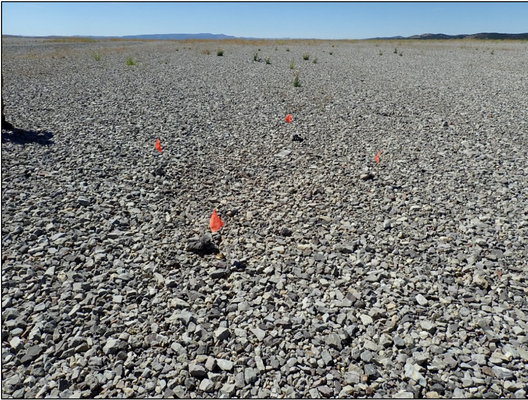
PL-9. Shallow Depression No. 2 on Disposal Cell Top Slope
