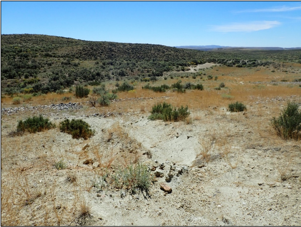
PL-21. Erosion Between Rock Berms West of Ancillary Cell
