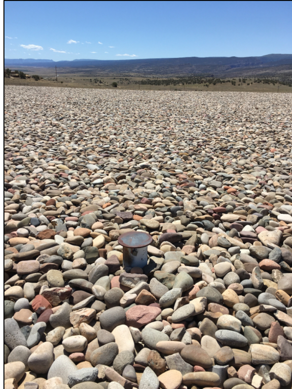
PL-4. Settlement Plate on Disposal Cell
