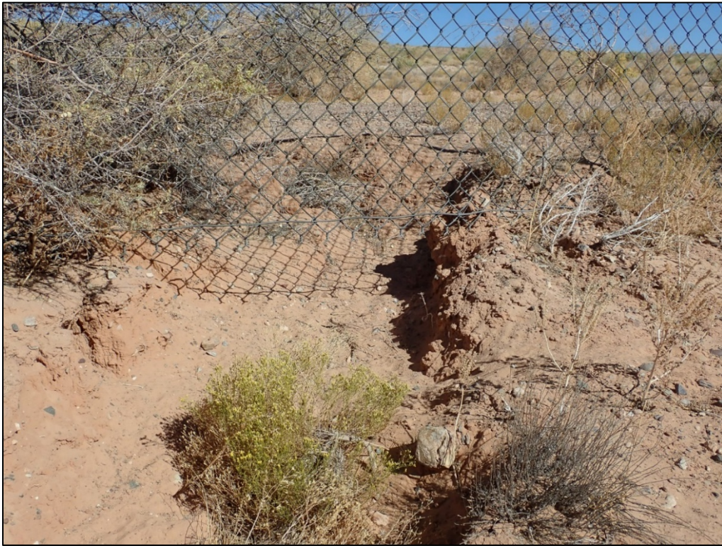
PL-3. Erosion Under Fence
