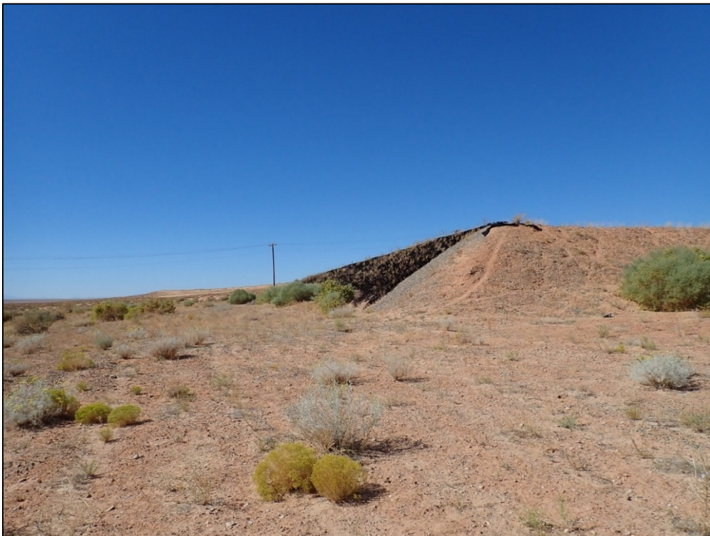
PL-10. Exposed Geofabric on South Side of Inactive, Lined Evaporation Pond
