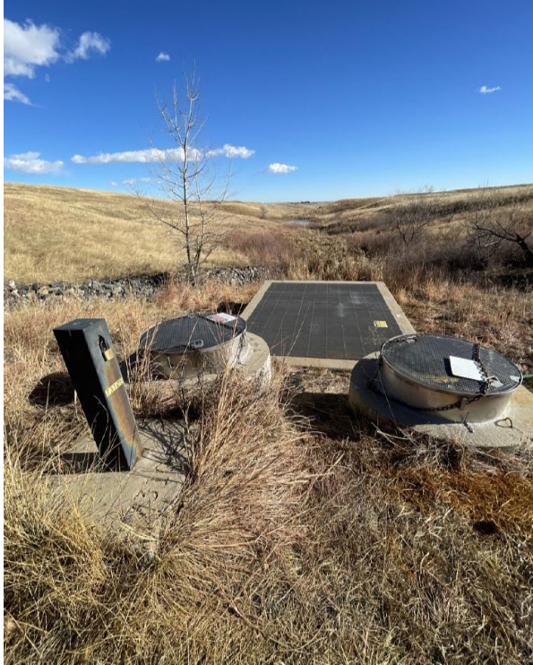
Present Landfill Treatment System
