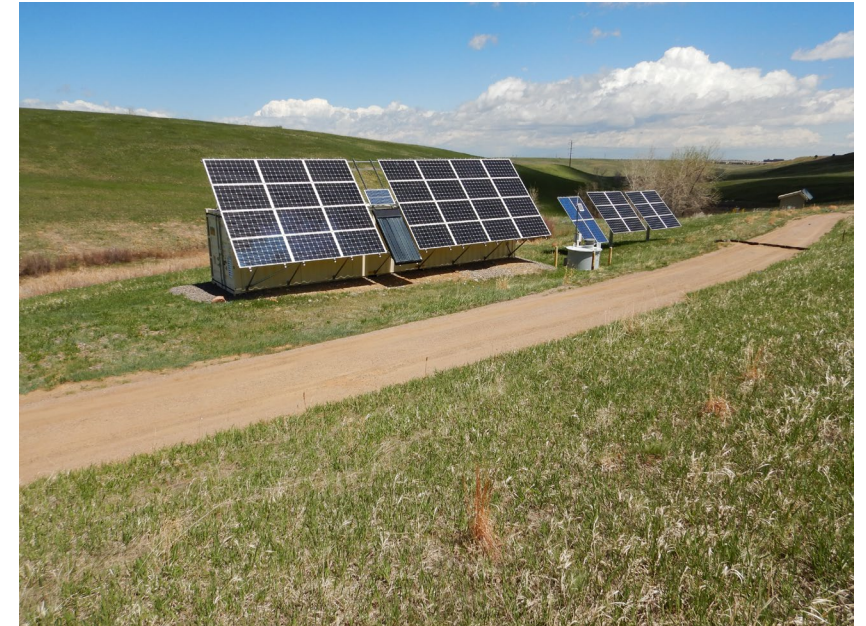
East Trenches Plume Treatment System
